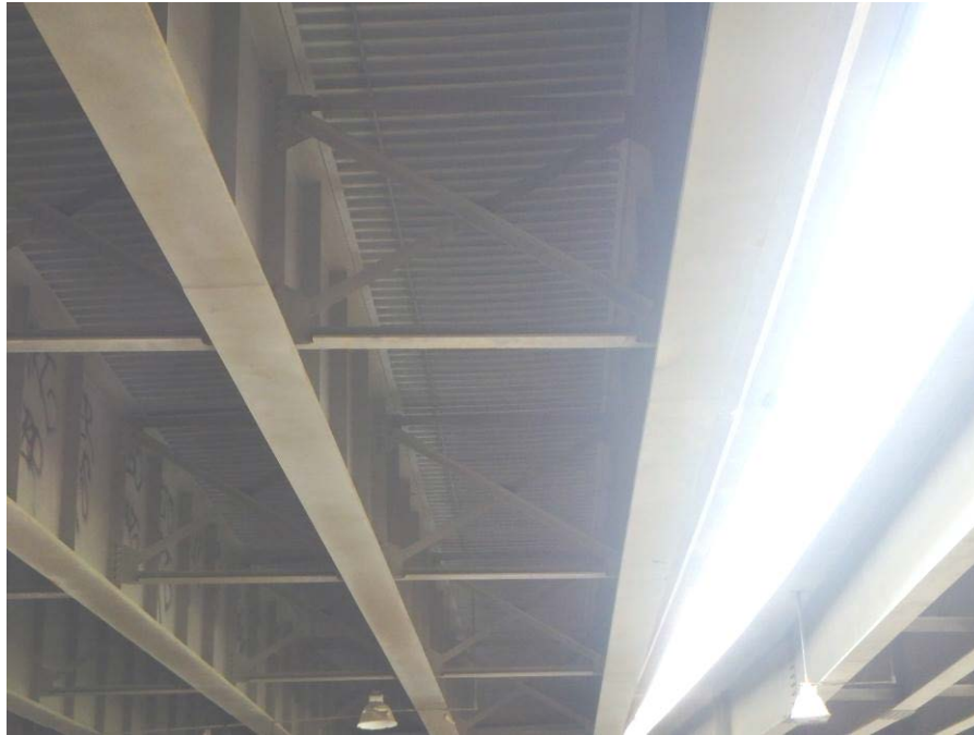
Photograph No. 33 – General View of Cross-Frames – Looking West in Bay 1 near the East Abutment
