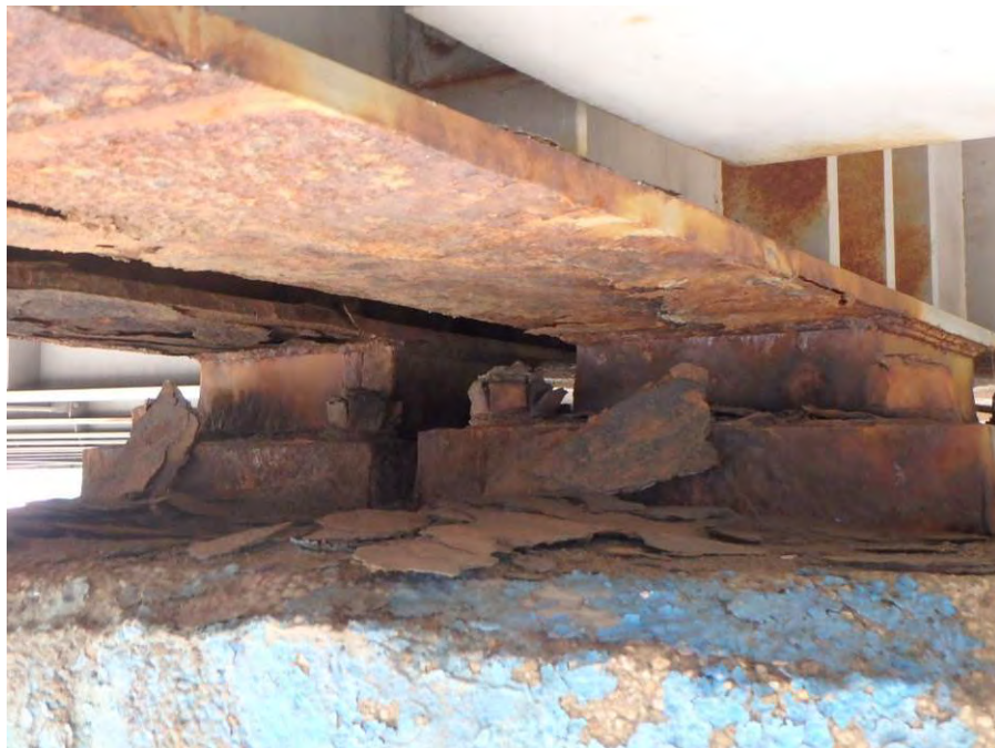
Photograph No. 46 – Moderate Section Loss in Bearing and Anchor Bolt Nuts of the Fixed Bearings at Column 4 of Bent 8, Looking Northwest
