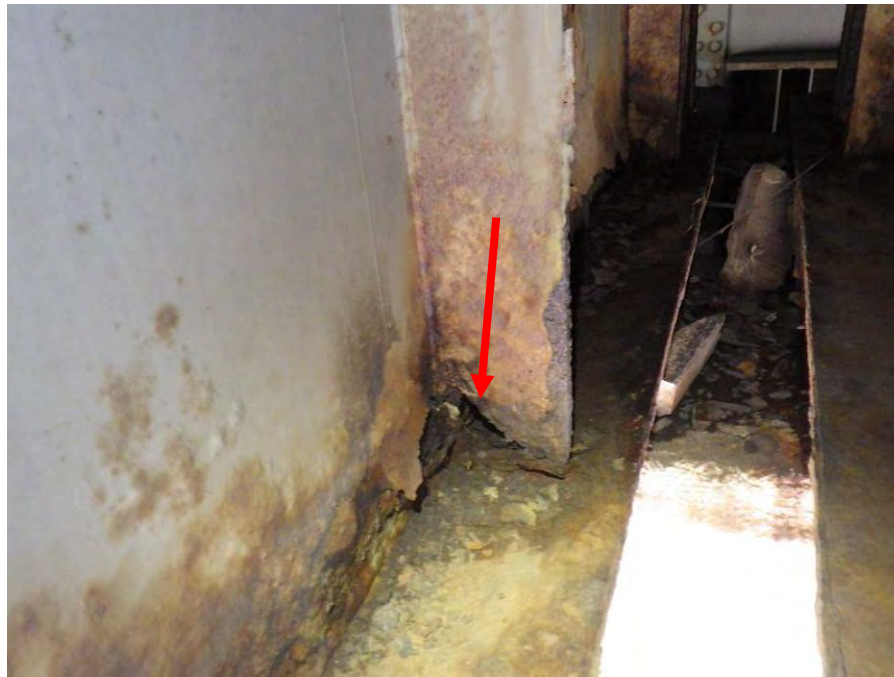
Photograph No. 10 – Active Up to 3" Diameter Corrosion Hole in West Cross Girder Stiffener at Bent 10 near Column 2
