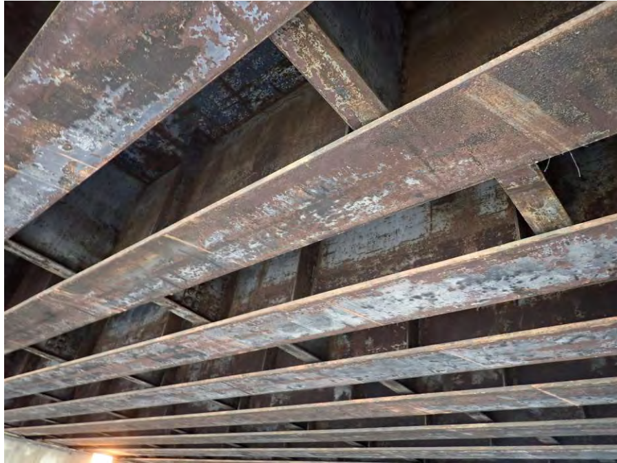
Photograph No. 7 – Typical Impact Scrapes on the Bottom Flanges of the Beams above the Center Lane, Looking Southeast
