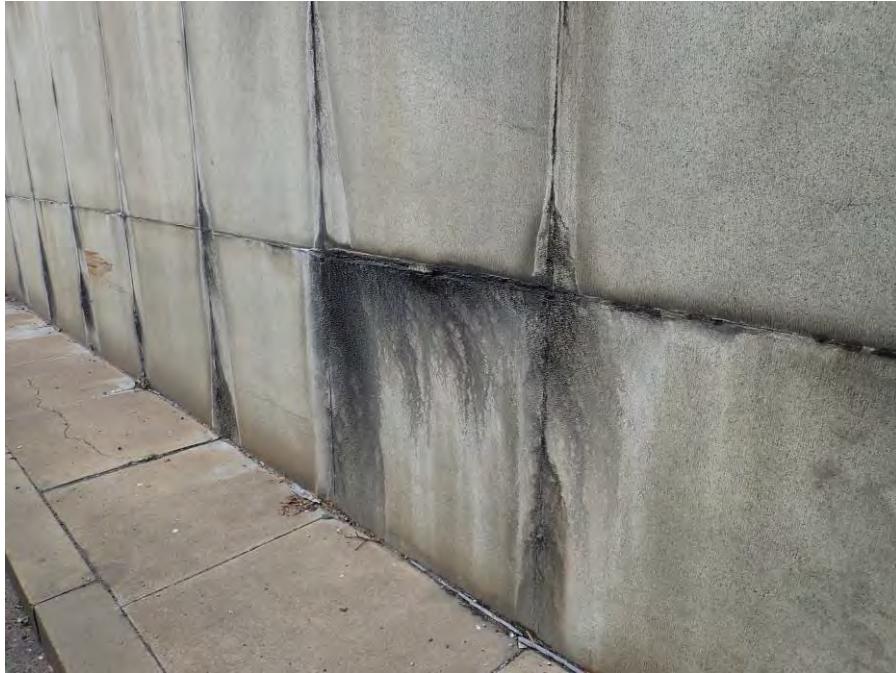
Photograph No. 21 – Southwest Wingwall. Note Mortar Cracking with Efflorescence
