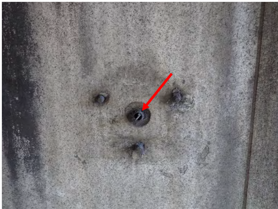
Photograph No. 34 – West Abutment Stem, Old Utility Conduit with Exposed Wiring
