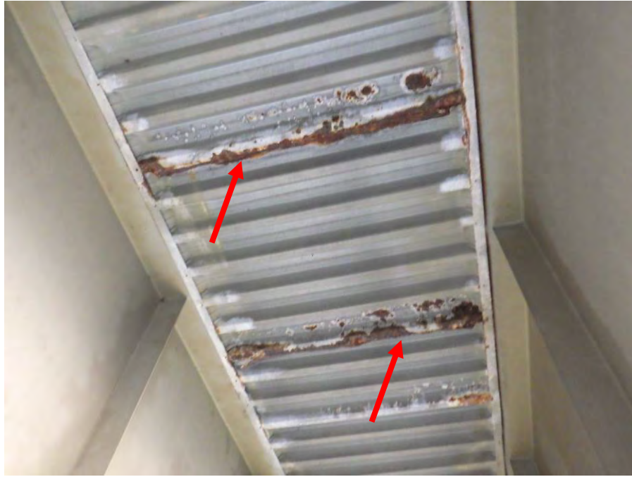
Photograph No. 15 – Minor Corrosion on Stay-In-Place Deck Forms in Bay 5 of Span 9
