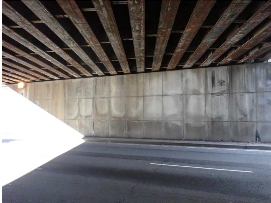
Photograph No. 11 – General View of the West Abutment. Note Typical Staining
