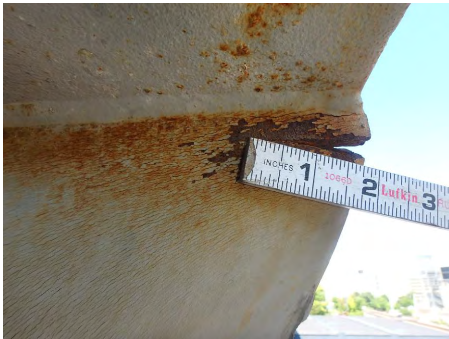
Photograph No. 52 – Girder 1, Span 4, Post-Tension Reinforcing System: 1 3/4" Long Crack in Vertical Portion of the 4 th Intermediate Support from the West
