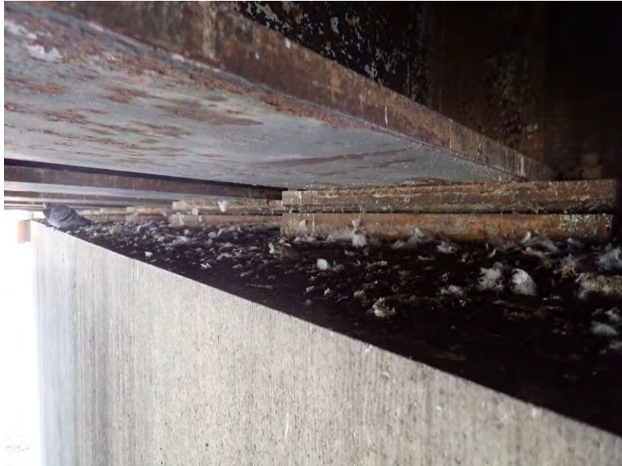
Photograph No. 27 – Typical Pigeon Debris on Both Bearing Seats – West Abutment Shown, Looking Southwest
