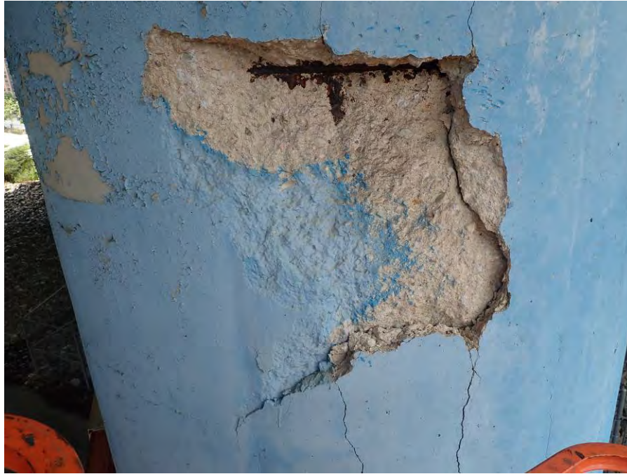
Photograph No. 67 – Bent 7, Column 1, 4'-0" Wide x 7'-0" High x Up to 4" Deep Spalled/Unsound Area with Exposed Corroded Reinforcing Steel in the North Face at the Top of the Column
