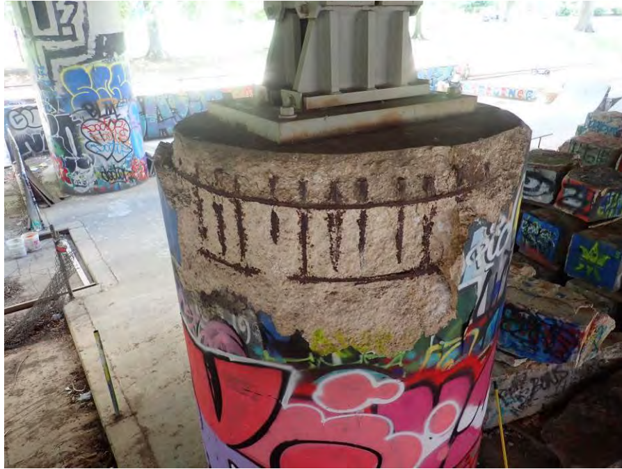
Photograph No. 69 – Bent 11, Column 1, South and West Faces – Unsound and Spalled Concrete with Exposed Corroded Reinforcing Steel
