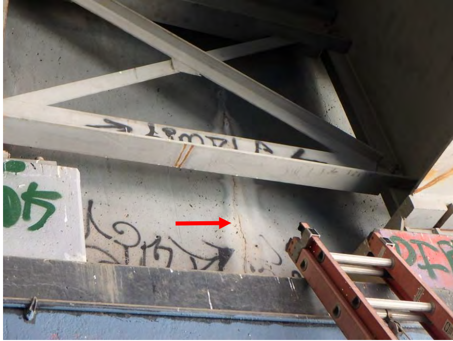
Photograph No. 71 – Typical Vertical Hairline Crack with Efflorescence in the East Abutment Backwall (Arrow), Bay 13 Shown
