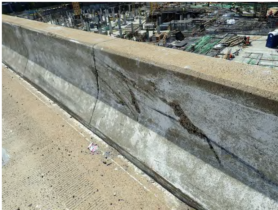
Photograph No. 20 – Minor Spalls, Scrapes and Gouges in the South Parapet – Span 4 Shown, Looking Southeast
