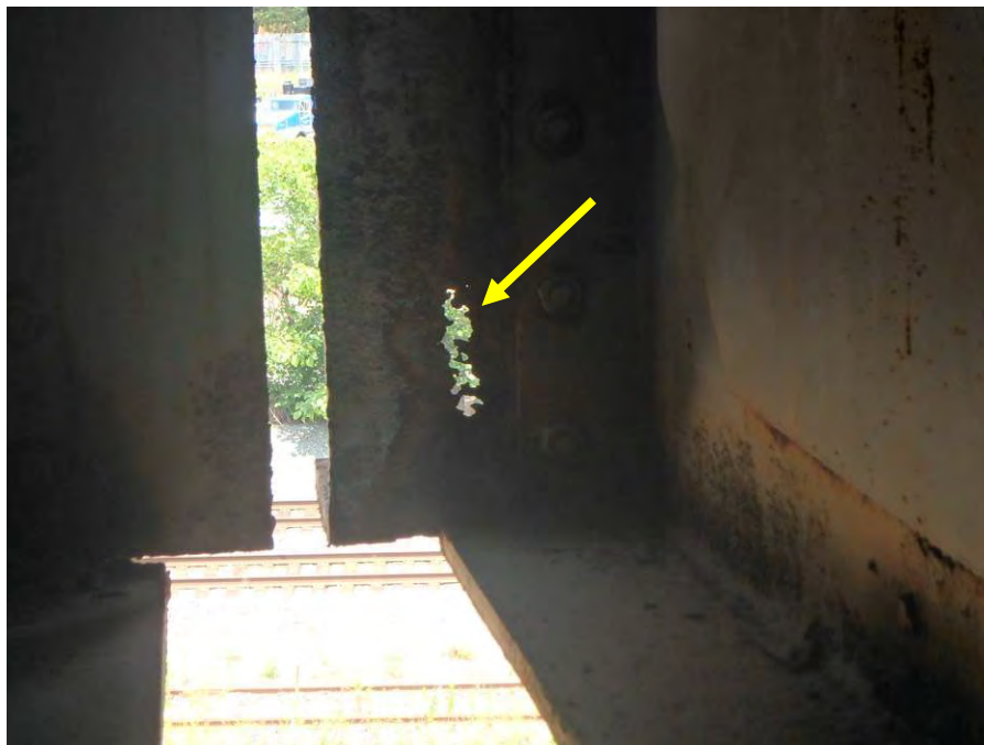
Photograph No. 38 – Corrosion Hole in the Web End of Girder 1 between the Cross Girders at Bent 4, Looking North
