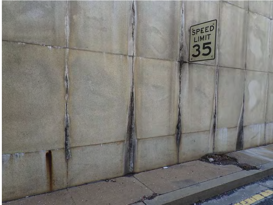
Photograph No. 19 – Southeast Wingwall. Note Mortar Cracking with Efflorescence
