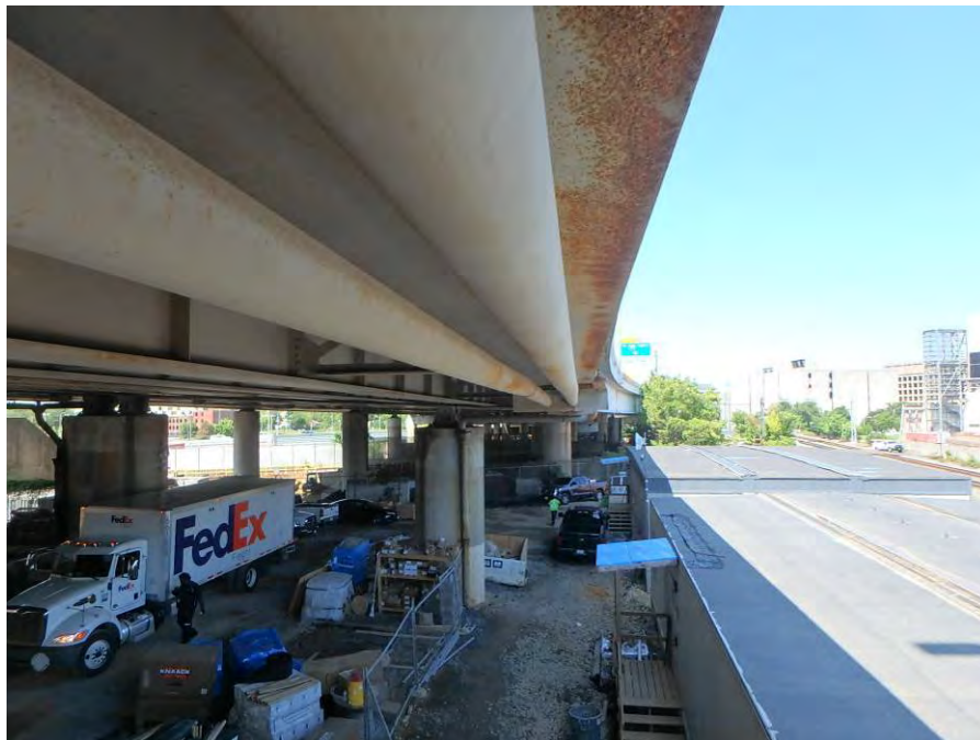
Photograph No. 50 – General View of a Post-Tensioning Retrofit – Span 4 Shown, Looking West
