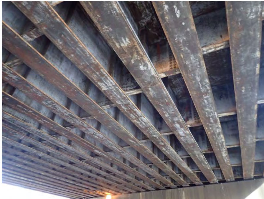
Photograph No. 6 – Typical Superstructure with Deteriorated Paint and Minor Corrosion
