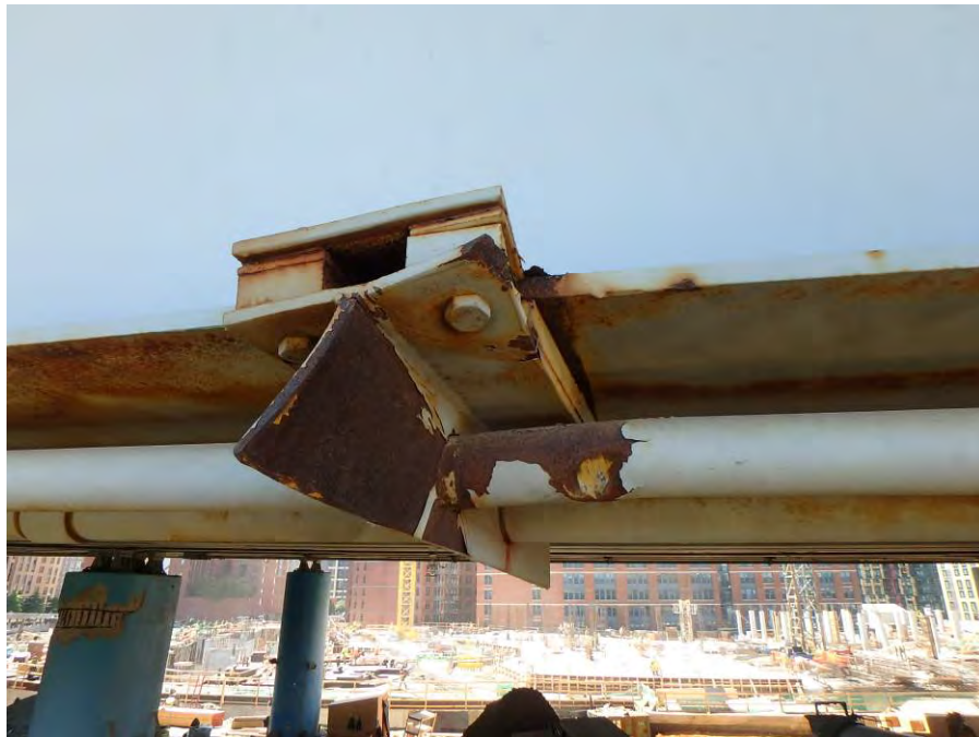
Photograph No. 54 – Impact Damage to the 3 rd Intermediate Support from the West of the Post-Tension Reinforcement on Girder 1 in Span 5. Note Damage to Rod Sheathing
