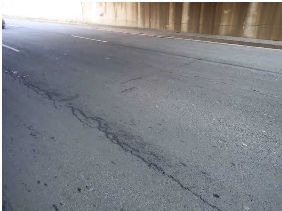
Photograph No. 30 – Up to 1/4" Wide Longitudinal Crack in the Right Lane of the Roadway below the Bridge
