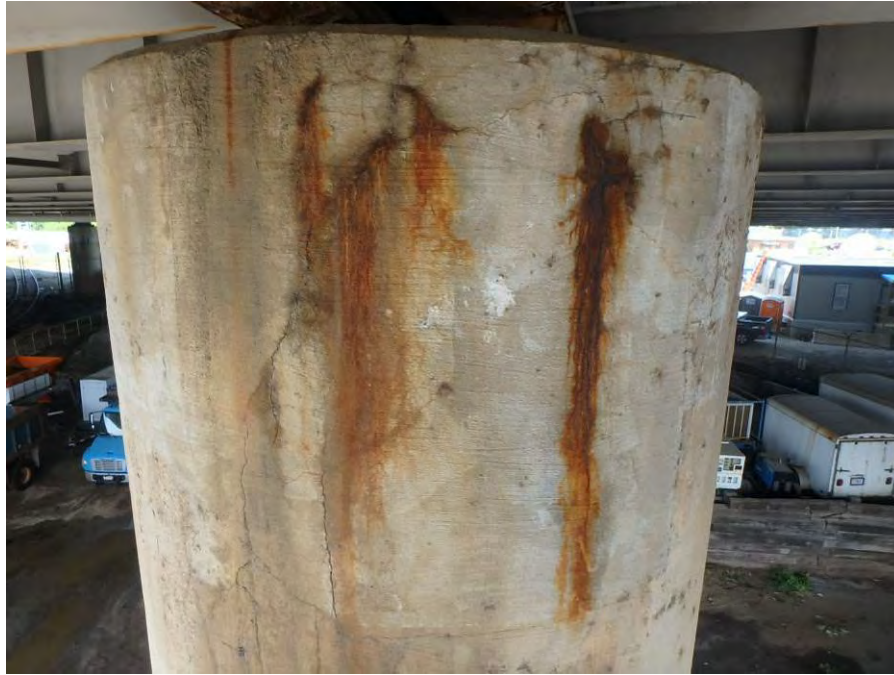
Photograph No. 61 – Bent 2, Column 4 – Cracking with Corrosion Staining near Top of Column
