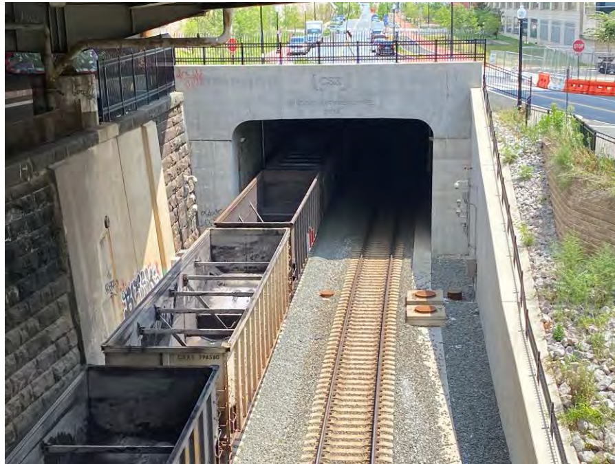
Photograph No. 12 – Looking Southeast from the Bridge at the CSX Railroad Tunnel near the East Abutment
