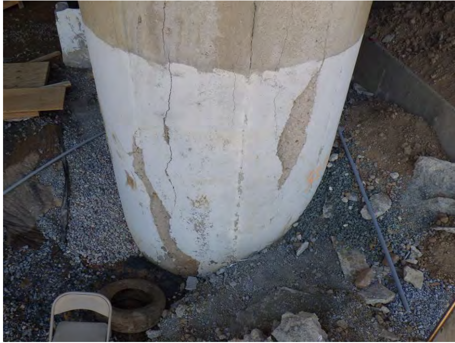
Photograph No. 63 – Bent 3, Column 3, South Face – 6'-0" High x 3'-0" Wide x Up to 2" Deep Spalled/Delaminated Area at Base
