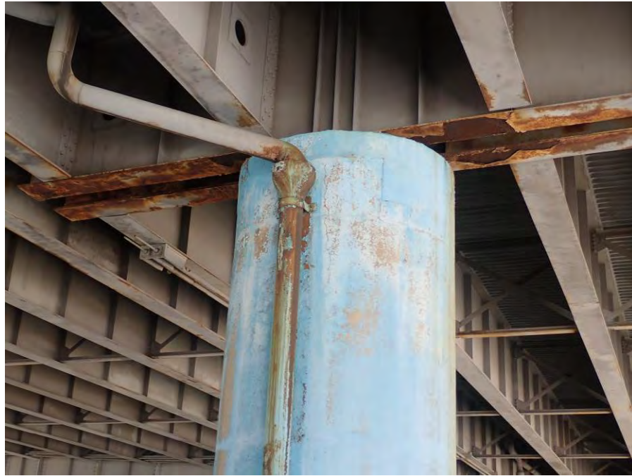
Photograph No. 6 – Moderate Corrosion on the Cross Girder Bottom Flanges at Column 3 of Bent 8
