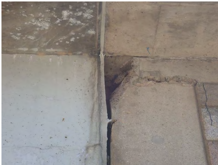
Photograph No. 74 – 18” High x 9” Wide x Up to 10” Deep Spall at the Top of the Southeast Wingwall
