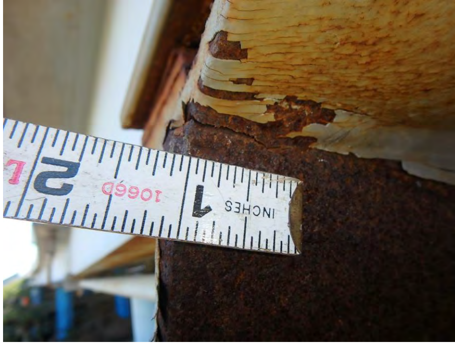
Photograph No. 55 – Girder 1, Span 5, Post-Tension Reinforcing System: 1 1/8" Long Crack in Vertical Leg of the 3 rd Intermediate Support from the West
