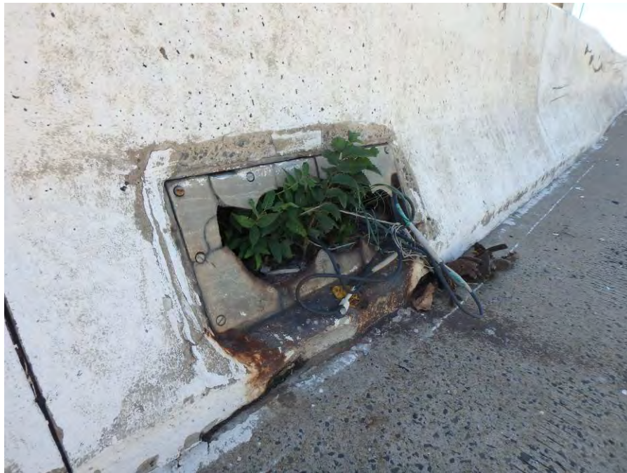
Photograph No. 78 – Span 10, Broken Electrical Access Panel Cover in the North Face of the Median Beneath the Eastbound Sign Structure
