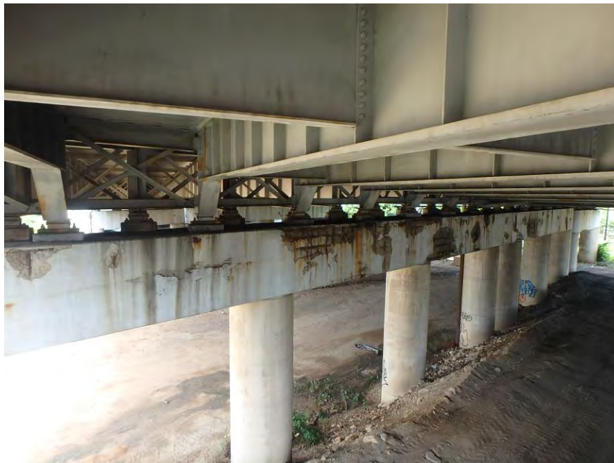
Photograph No. 56 – East Face of the West Pier with Numerous Cracks and Spalls with Exposed Corroded Reinforcing Steel
