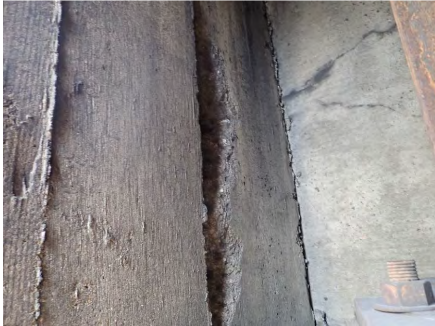
Photograph No. 25 – 2'-4" High x 6" Wide x Up to 3 3/4" Deep Spall in the South Face of the Northeast Wingwall
