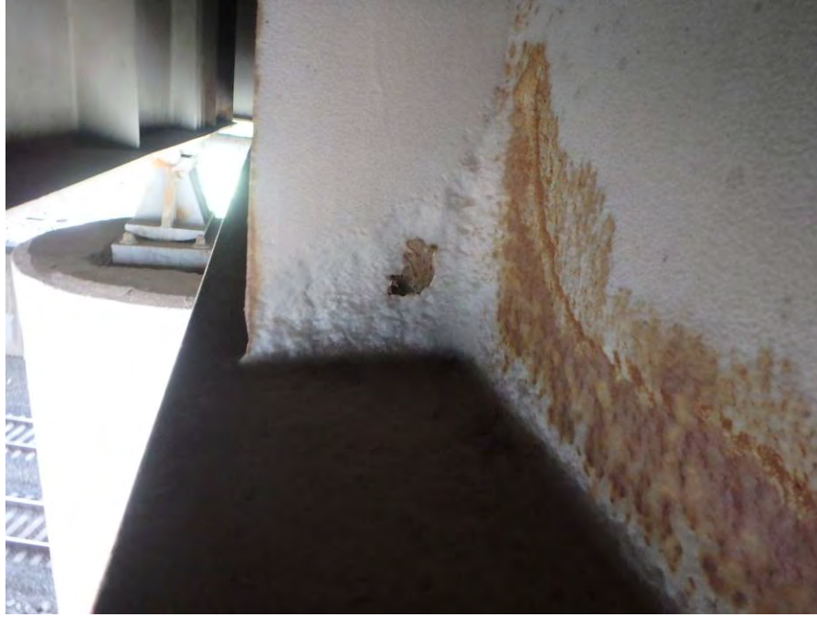
Photograph No. 9 – Corrosion Hole in the Base of the East Cross Girder Stiffener (West Face) at Bent 9 near Column 3. Note Section Loss in the Girder Web
