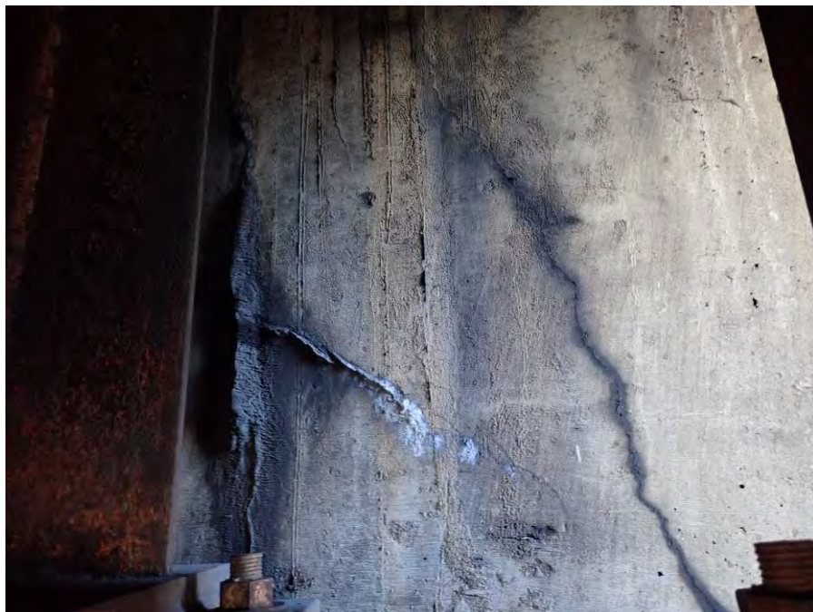
Photograph No. 22 – Typical Hairline Cracks in the West Abutment Backwall. Bay 1 Shown
