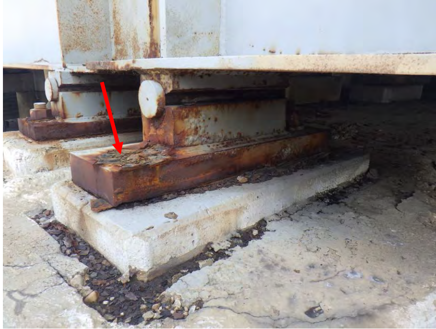
Photograph No. 43 – Fixed Bearing Anchor Bolt for Girder 20 at the West Pier is Broken/Missing (Arrow)
