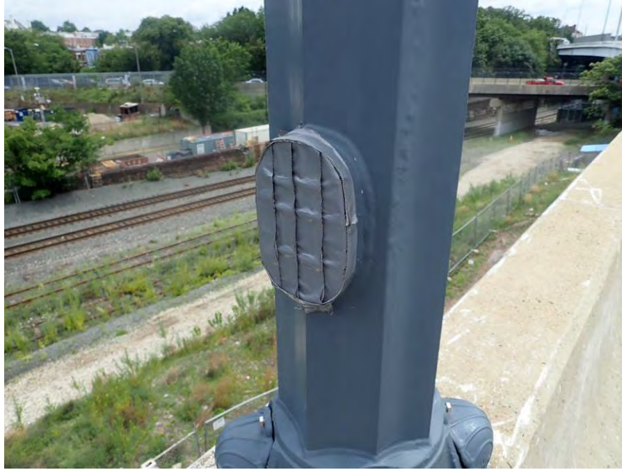
Photograph No. 79 – North Light Standard in Span 4 – Duct Tape Used to Cover Handhole Opening
