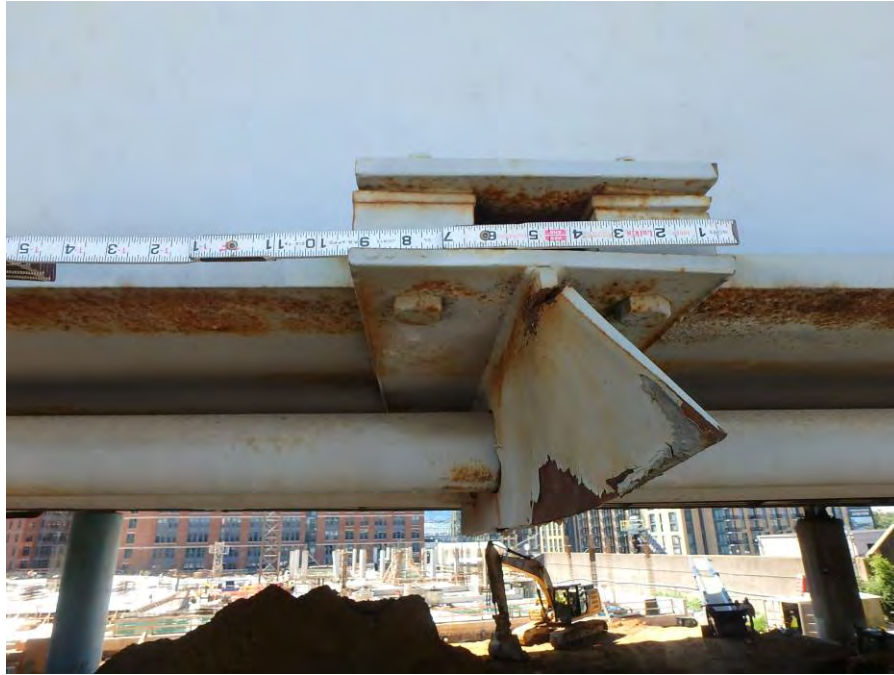
Photograph No. 51 – Post-Tension Reinforcement on Girder 1 in Span 4 – Impact Damage to the 4 th Intermediate Support from the West End
