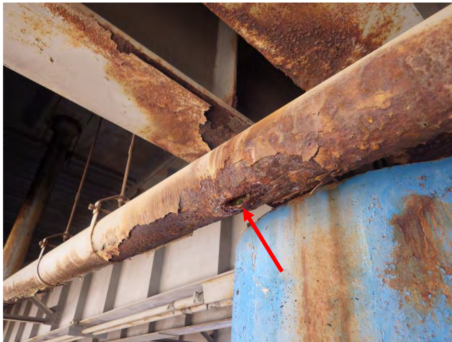
Photograph No. 30 – Minor to Severe Corrosion in the Horizontal Drain Pipe at Bent 4, Column 2 with a 6" Long x 2" Wide Corrosion Hole, Looking Northwest
