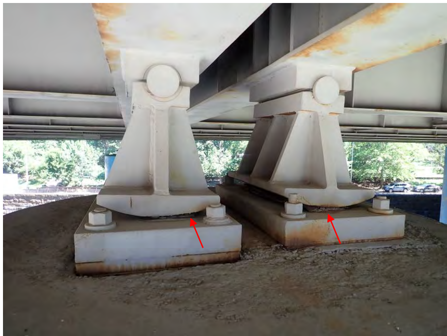
Photograph No. 42 – Bent 7, Typical Painted Over Crevice Corrosion Possibly Restricting Normal Rotation of Bearings
