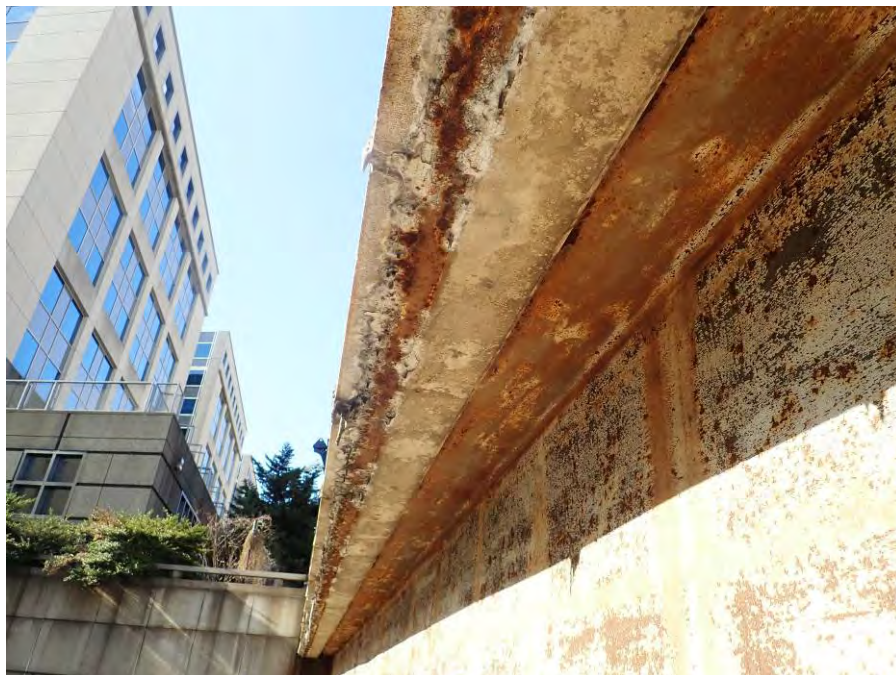
Photograph No. 8 – South Fascia. Note Efflorescence and Stalactites
