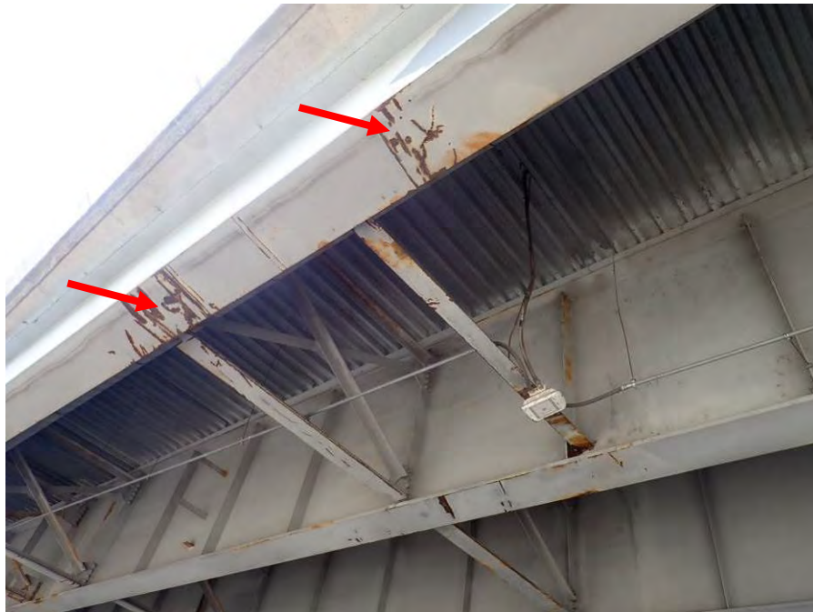
Photograph No. 80 – Typical LED Light Fixture in Span 7 above New Jersey Avenue. Note Impact Marks to Underside of Longitudinal Girder (Arrows)
