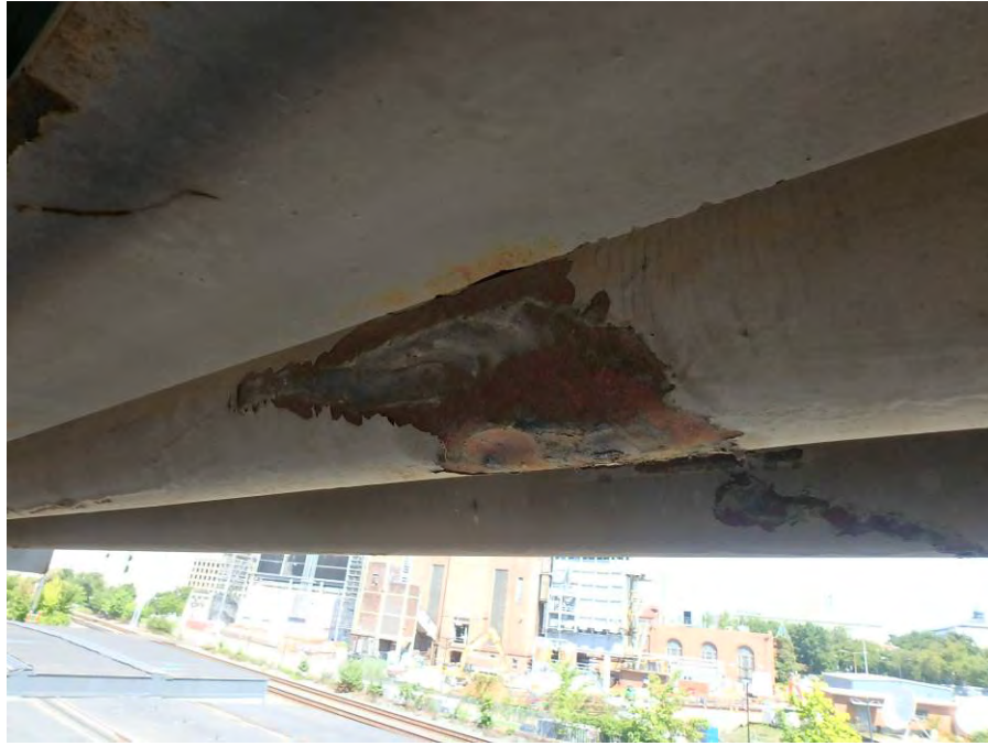
Photograph No. 53 – Girder 1, Span 4, Post-Tension Reinforcing System: Impact Damage to Sheathing
