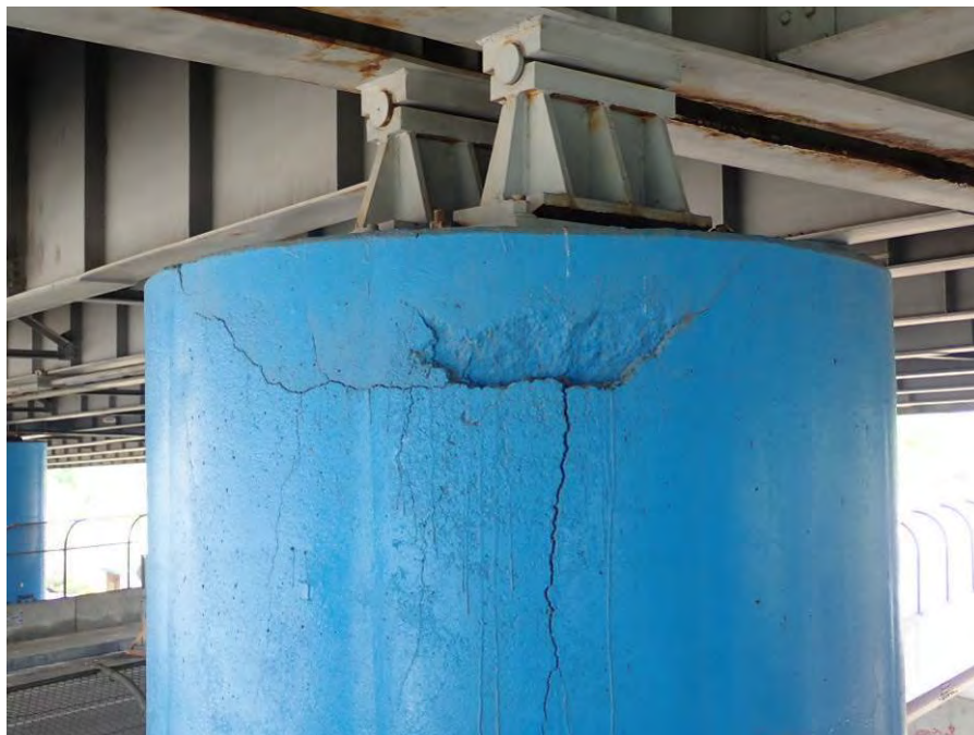
Photograph No. 68 – Bent 7, Column 3, Southeast Face – Area of Unsound Concrete with a 24" Wide x 7" High x 3" Deep Spall
