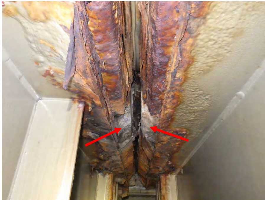
Photograph No. 16 – Moderate Corrosion of the Bent 10 Joint under the Eastbound Lanes. Note the Spalls in Each Side of the Joint (Arrows)
