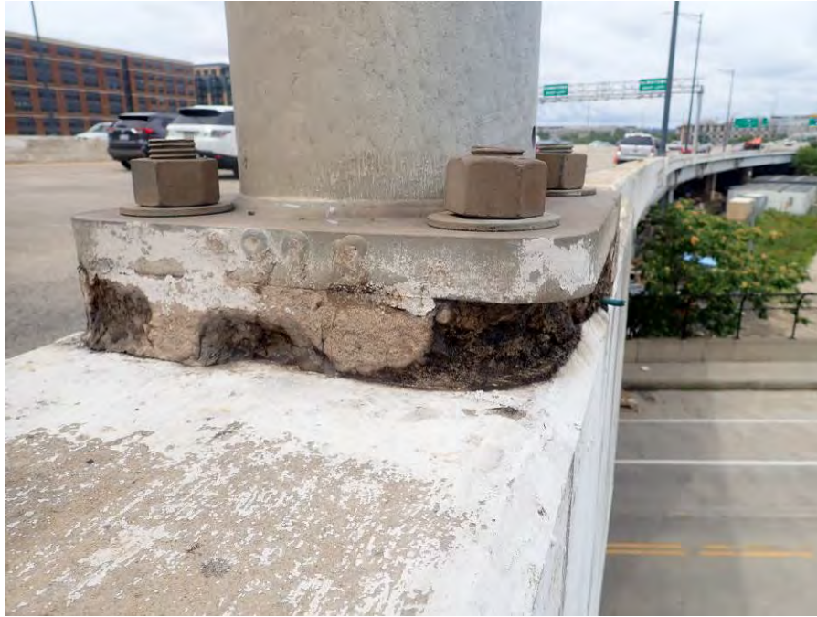
Photograph No. 23 – Up to 1” Deep Moderate Scaling in the Sign Structure Column Base Mortar on the Westbound North Parapet in Span 7
