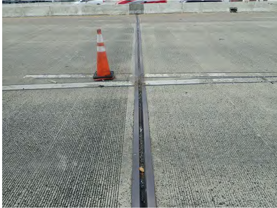
Photograph No. 19 – Typical Deck Joint with Minor to Moderate Debris Accumulation in Seal, Westbound Lanes at Bent 7 Shown, Looking South
