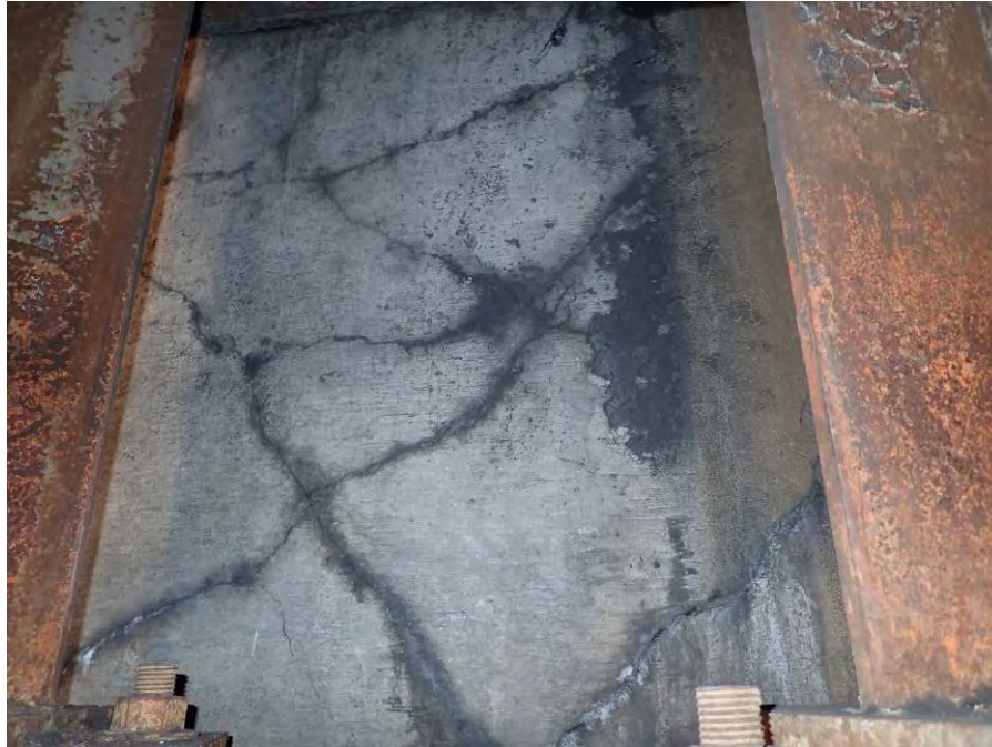
Photograph No. 23 – Diagonal Hairline Cracks in the East Abutment Backwall. Bay 1 Shown
