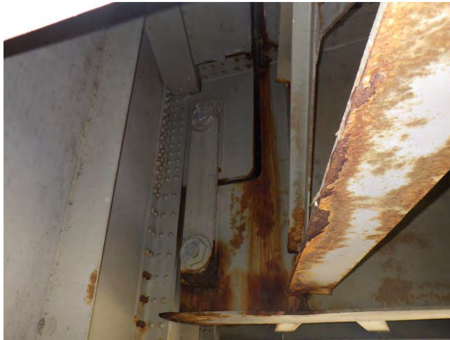
Photograph No. 14 – Minor Corrosion on the Pin and Hanger Assembly at Girder 6 in Span 9, Looking South
