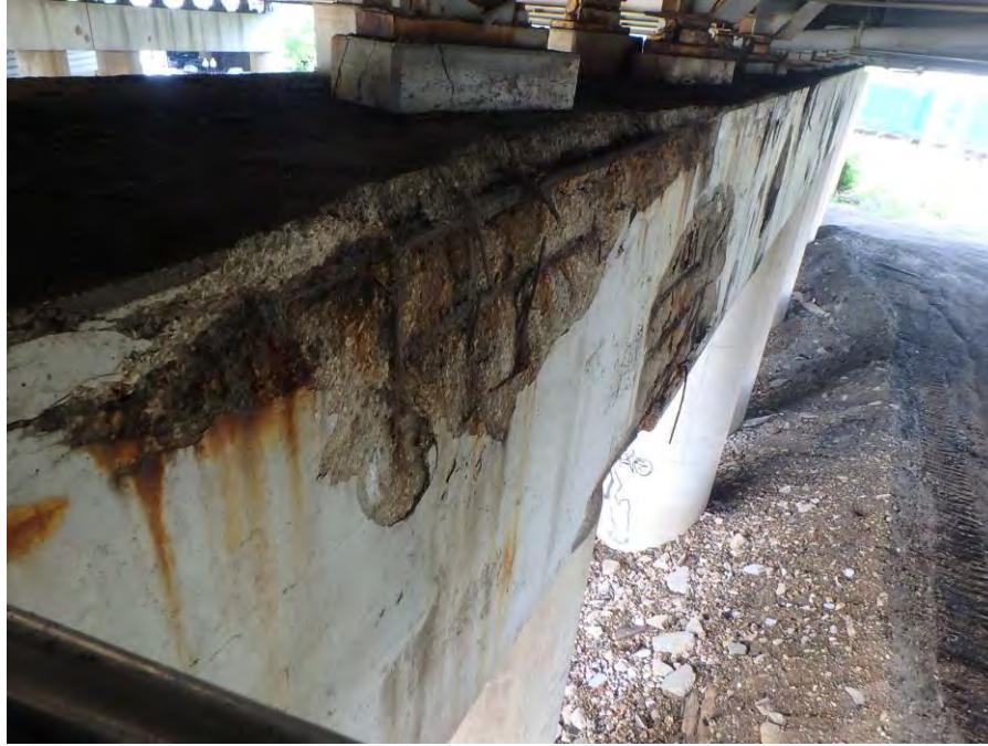
Photograph No. 59 – Spalls with Exposed Corroded Reinforcing Steel in the East Face of the West Pier below Girders 15 through 17, Looking Northwest
