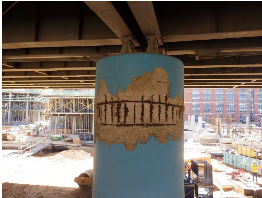
Photograph No. 66 – Bent 5, Column 2, North Face – 5’-0” High x 12’-0” Wide x Up to 4” Deep Area of Spalled/Delaminated Concrete with Exposed Corroded Reinforcing Steel
