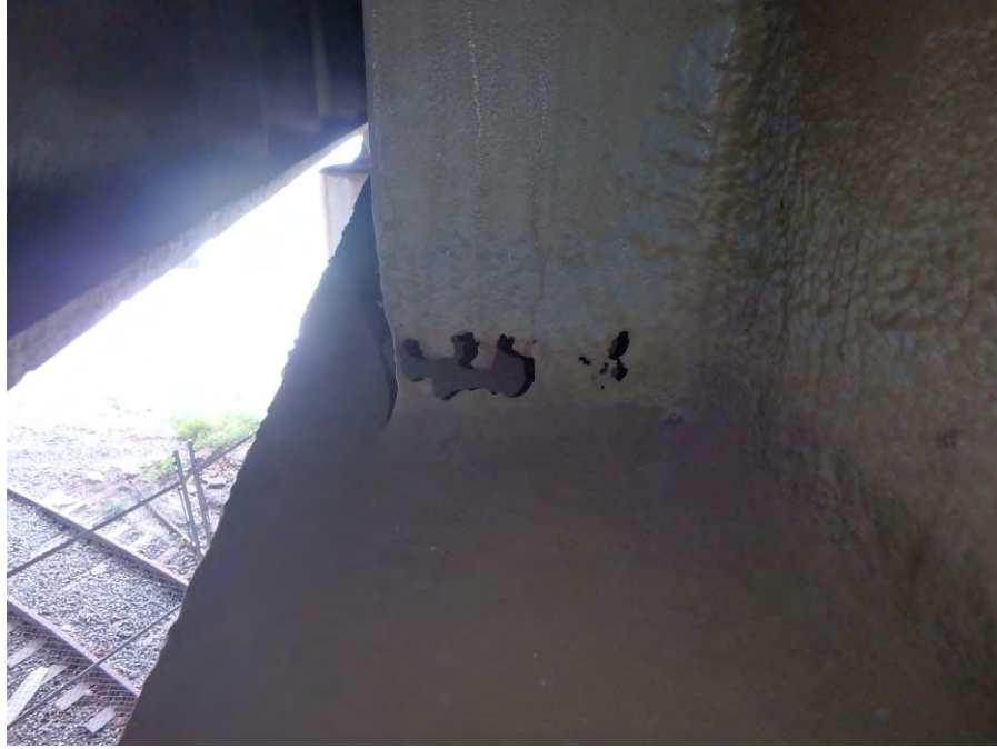
Photograph No. 5 – Two Corrosion Holes (1/2" x 1" and 2 1/2" x 1") at the Base of the East Cross Girder Stiffener at Bent 1
