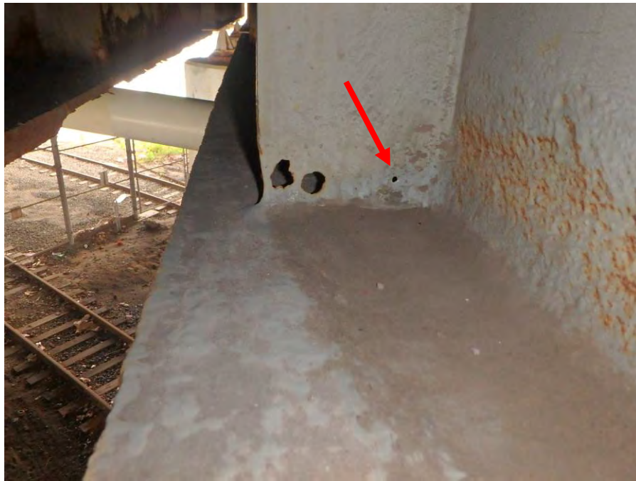
Photograph No. 4 – Two 1" Diameter Corrosion Holes and a 3/16" Diameter Corrosion Hole (Arrow) in a West Cross Girder Stiffener at Bent 1 near Column 3. Note Section Loss in Girder Web
