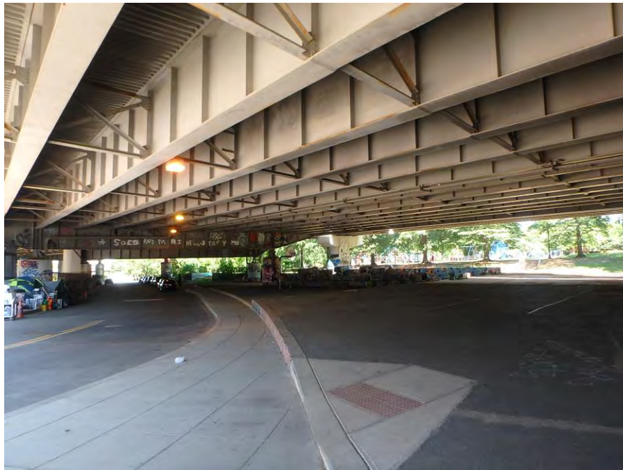
Photograph No. 32 – General View of the Superstructure – Looking Northwest in Span 12 Shown
