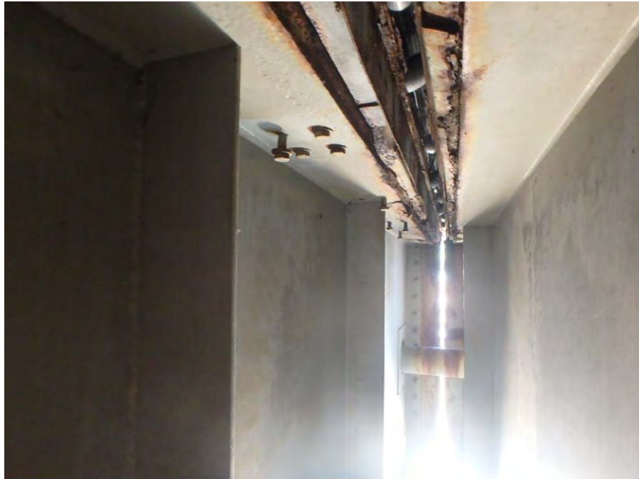
Photograph No. 2 – Typical Abandoned Joint Attachment Fasteners, Cross Girder at Bent 2 Shown
