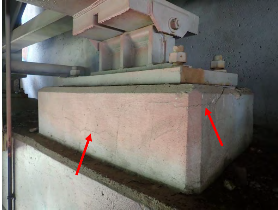
Photograph No. 73 – Typical Hairline Cracks in Concrete Repairs to East Abutment Pedestals (Arrows) – West Side of Girder 2 Shown
