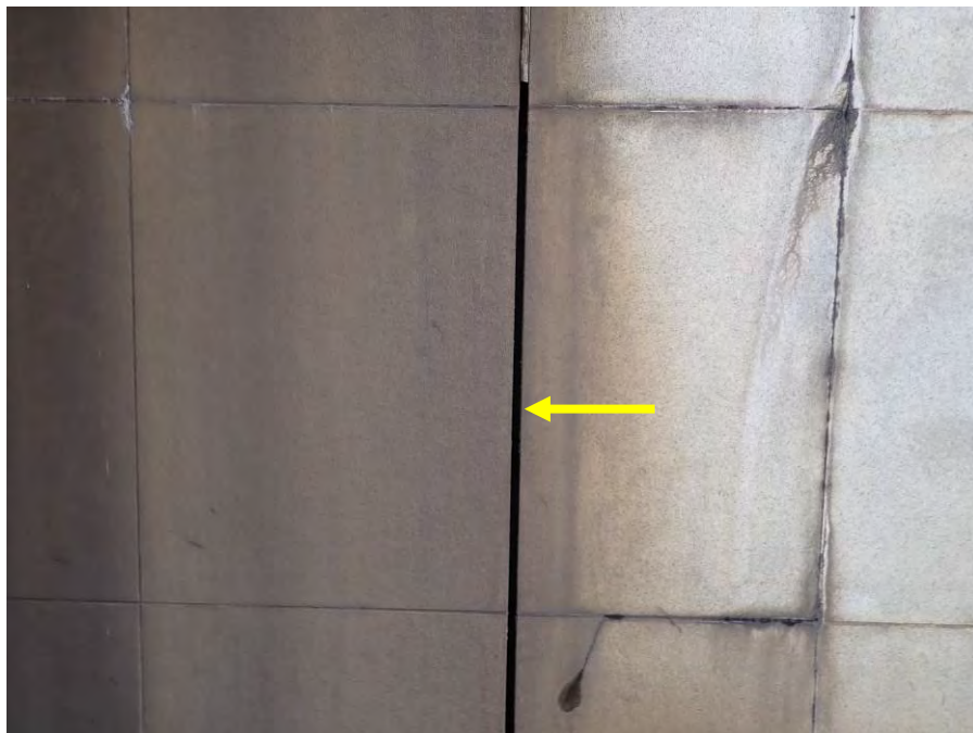
Photograph No. 26 – Typical Missing/Deteriorated Abutment to Wingwall Joint Material. Southeast Wingwall Shown
