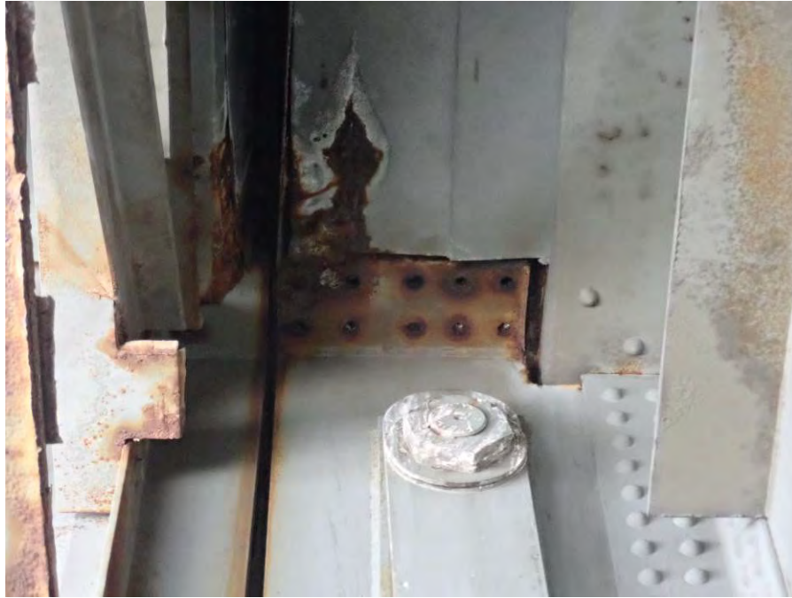
Photograph No. 37 – Girder Top Flange Connection Fasteners Missing above the Pin and Hanger Connections – Girder 16 at Bent 11 Shown, Looking North
