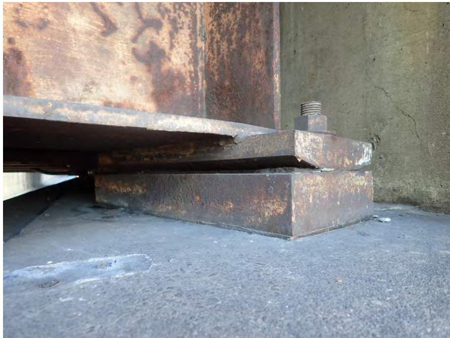
Photograph No. 10 – Typical West Abutment Bearing. Note Deteriorated Paint and Minor Corrosion. Bearing 1 Shown
