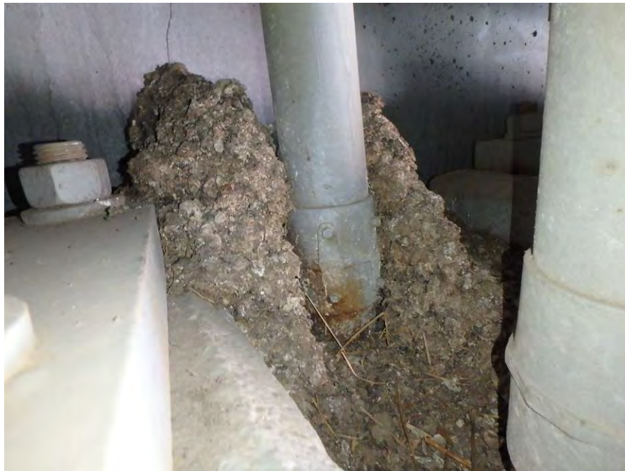
Photograph No. 72 – Significant Debris Accumulation on the East Abutment Bridge Seat in Bay 8
