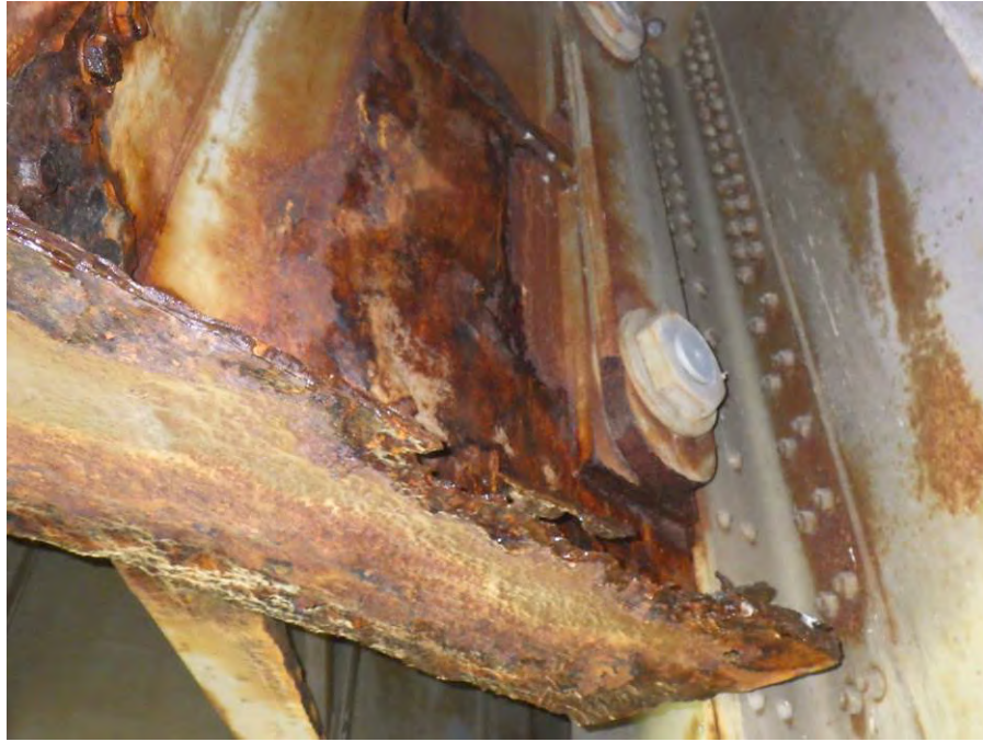
Photograph No. 41 – Bent 10A, South Side of Girder 4, Severe Section Loss for the Full-Width of the Girder Bottom Flange
