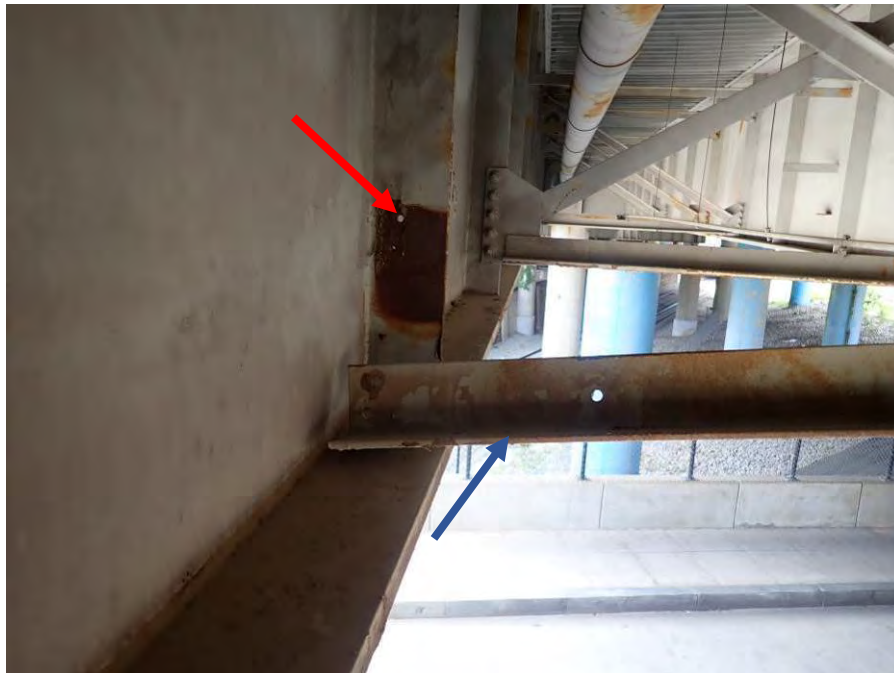
Photograph No. 40 – Location of Missing Fasteners (Red Arrow) at Displaced Horizontal Light Fixture Support between Girders 1 and 2 in Span 7 above New Jersey Avenue
