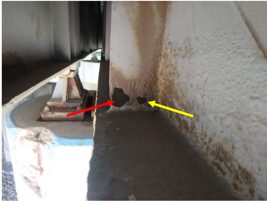
Photograph No. 8 – 3" Diameter (Red Arrow) and 1" Diameter (Yellow Arrow) Corrosion Holes in the Base of the East Cross Girder Stiffener (West Face) at Bent 9 near Column 4
