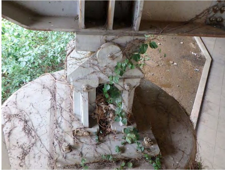
Photograph No. 47 – Overgrown Vegetation on Bearing 1 at Bent 9A
