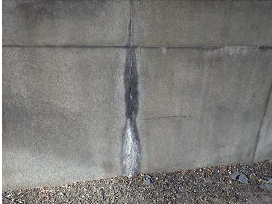
Photograph No. 17 – Cracked Mortar with Efflorescence in the West Abutment Stem
