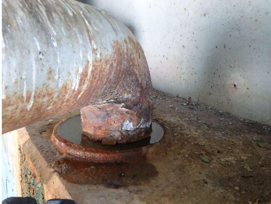
Photograph No. 75 – Clogged Drain Pipe at the South End of the East Abutment
