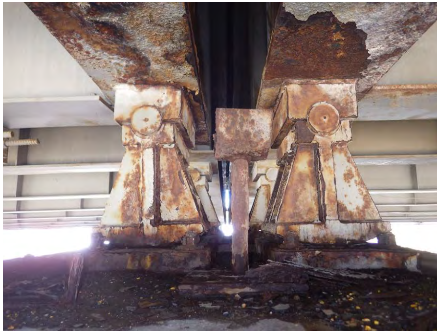
Photograph No. 44 – Moderate Section Loss on Bearing and Anchor Bolt Nuts of the Rocker Bearings (Column 2 of Bent 3 Shown, Looking North)
