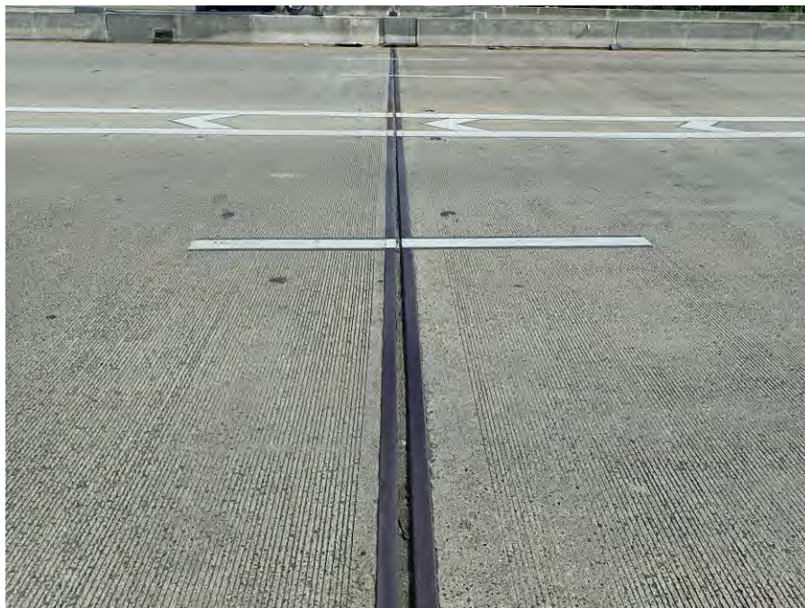
Photograph No. 18 – Typical Deck Joint with Minor to Moderate Debris Accumulation in Seal, Eastbound Lanes at Bent 1 Shown, Looking North
