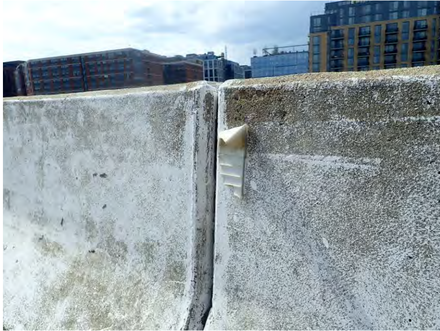
Photograph No. 21 – Typical Broken Reflector Attached to Parapets and Median (South Parapet in Span 1 Shown, Looking Southeast)
