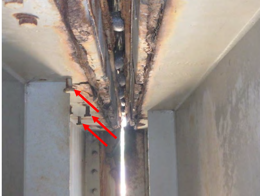
Photograph No. 17 – Typical Area of Moderate Corrosion and Evidence of Moisture Leakage – Bent 2 Joint Shown. Note Abandoned Joint Attachment Fasteners (Arrows)
