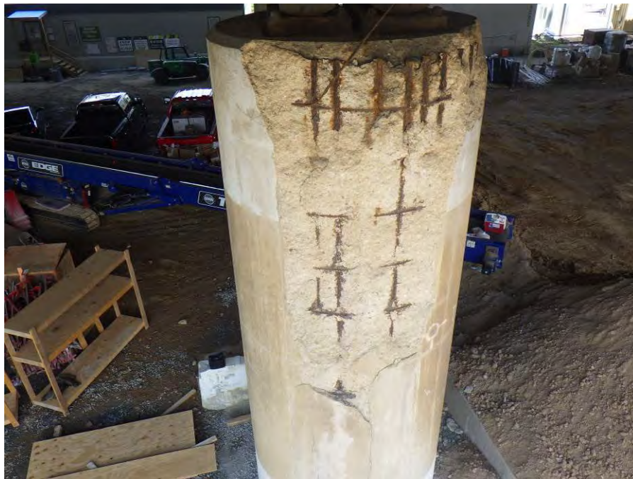
Photograph No. 62 – Bent 3, Column 3, South Face – Up to 3'-0" Wide x 10'-0" High x Up to 8" Deep Spall/Delamination with Exposed Corroded Reinforcing Steel
