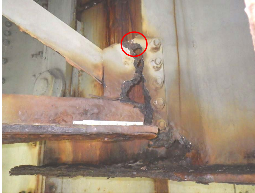
Photograph No. 35 – Cross-Frame Connection to the North Side of Girder 4 at Bent 9A – Significant Section Loss with Only 7/8” of Connection Remaining (Encircled). Note 5” Wide x 2” High Hole at Bottom of Stiffener
