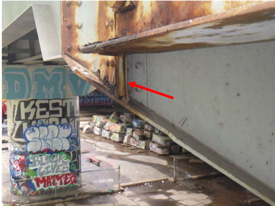
Photograph No. 12 – 1/4" Crevice Corrosion at Bottom of Stiffener at Connection to Girder 1 at Bent 10 in Span 10A
