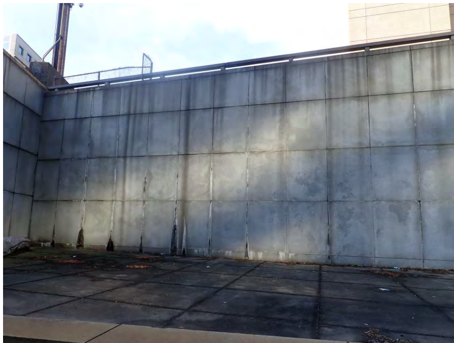
Photograph No. 20 – Northwest Wingwall. Note Mortar Cracking with Efflorescence
