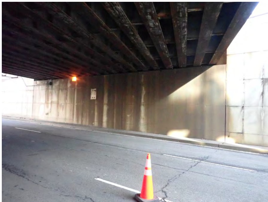
Photograph No. 12 – General View of the East Abutment. Note Typical Staining
