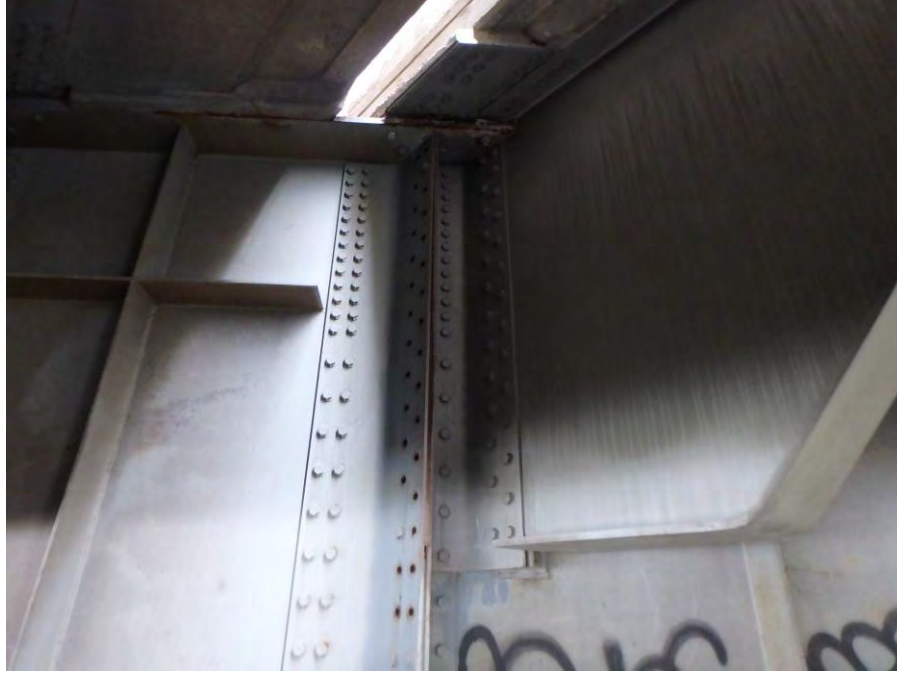
Photograph No. 11 – 29 Fasteners Missing in Stiffener North of Girder 1 at Bent 10
