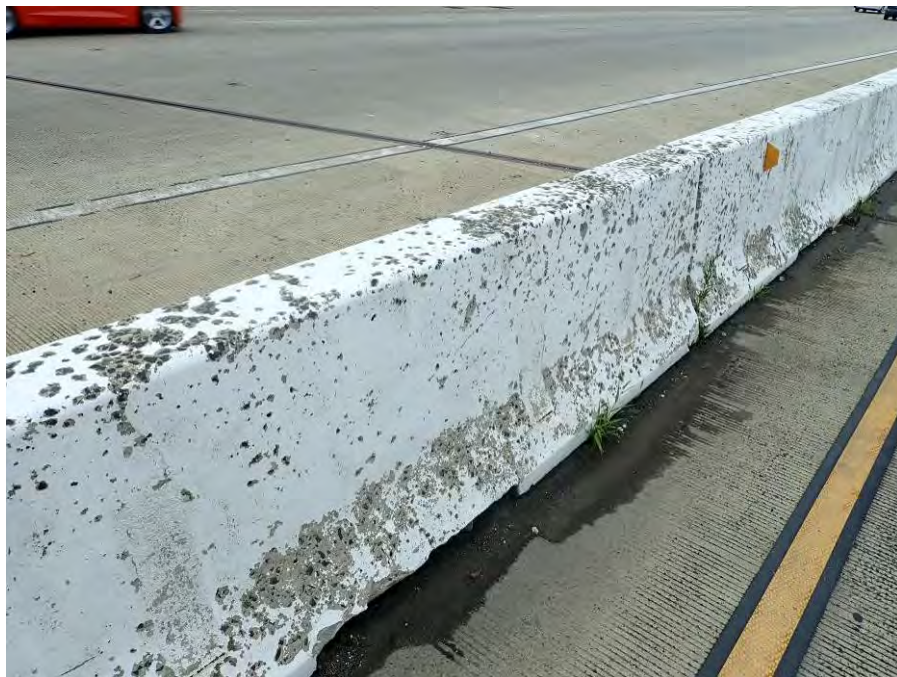
Photograph No. 22 – Paint Deterioration on South Barrier of the North Ramp Section in Span 10, Looking Southwest
