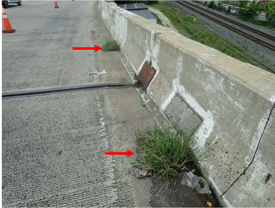
Photograph No. 27 – Typical Clogged Scuppers – Spans 5 and 6 in the Westbound Lanes Shown, Looking West
