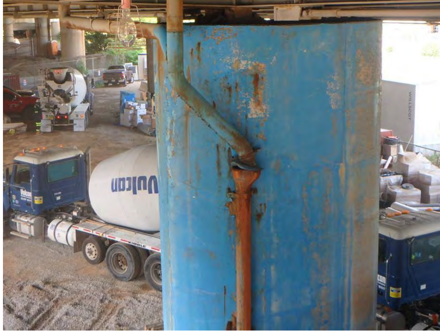
Photograph No. 29 – Typical Downspout Exhibiting Corrosion Staining with Corrosion Visible where Paint has Failed
