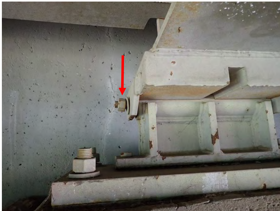
Photograph No. 48 – Bearing 3 at the East Abutment – Loose Shoulder Rod with South Nut Backed Off 3/4" – North Nut Shown
