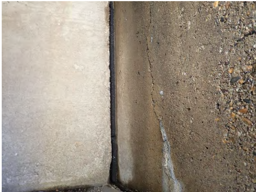
Photograph No. 24 – 1/4" Wide Vertical Crack in the North Face of the Southeast Wingwall adjacent to the East Abutment Backwall
