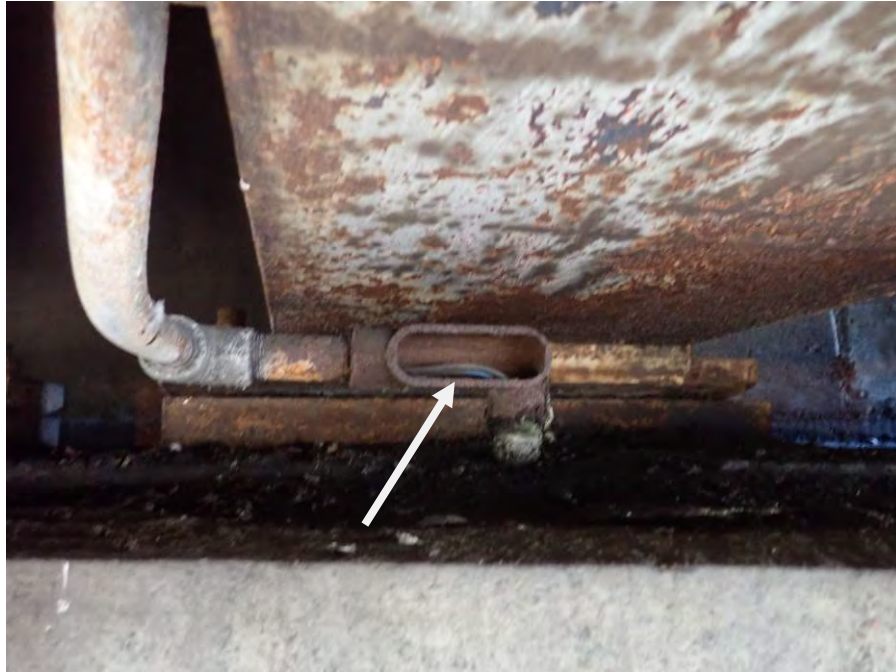
Photograph No. 33 – Missing Conduit Junction Box Cover Exposing Wiring at Bearing 3 on the West Abutment (Arrow)
