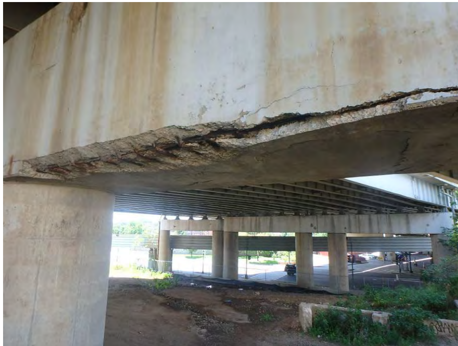
Photograph No. 58 – 14'-6” Wide x 12” High x 3'-0” Under Delamination/Spall with Exposed Corroded Reinforcing Steel and a 1/8” Wide Horizontal Crack in the West Pier Cap at the North Ramp Section
