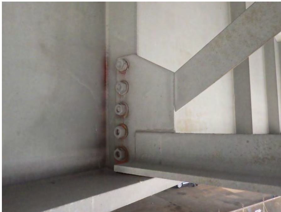
Photograph No. 36 – Five Loose Bolts and Up to 7/8” Gap between Connection Plate and Stiffener of Cross-frame Connection on South Side of Girder 18 at Mid-span of Span 11
