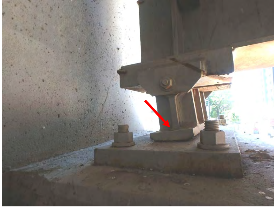
Photograph No. 49 – Bearing 15 at the East Abutment – North Anchor Bolt Broken/Missing (Arrow) and Bearing Leaning Excessively to the East
