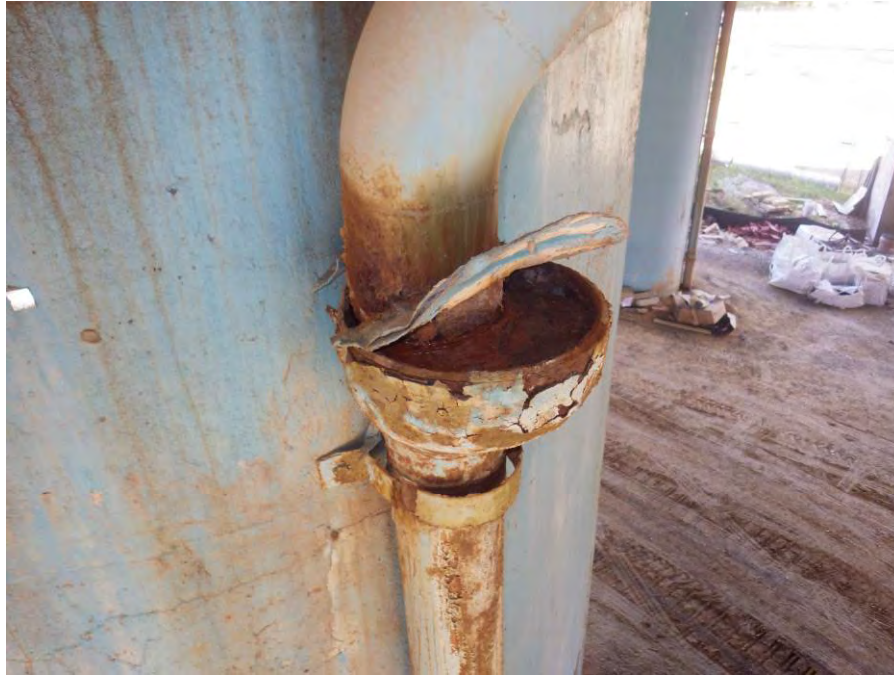
Photograph No. 31 – Downspout at Bent 5, Column 2 Completely Clogged with Debris
