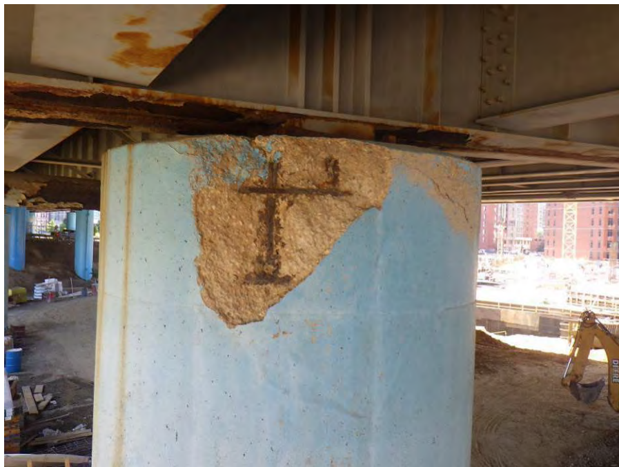
Photograph No. 64 – Bent 4, Column 1, West Face – Unsound /Spalled Area of Concrete at the Top of the Column
