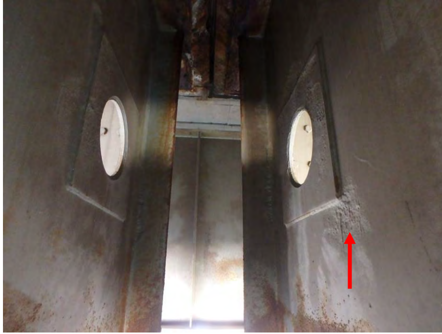
Photograph No. 3 – Typical Welded Plates at Location of Old Scupper Drain Pipe. Note Section Loss in Cross Girder Webs adjacent to the Welded Plates (Arrow)
