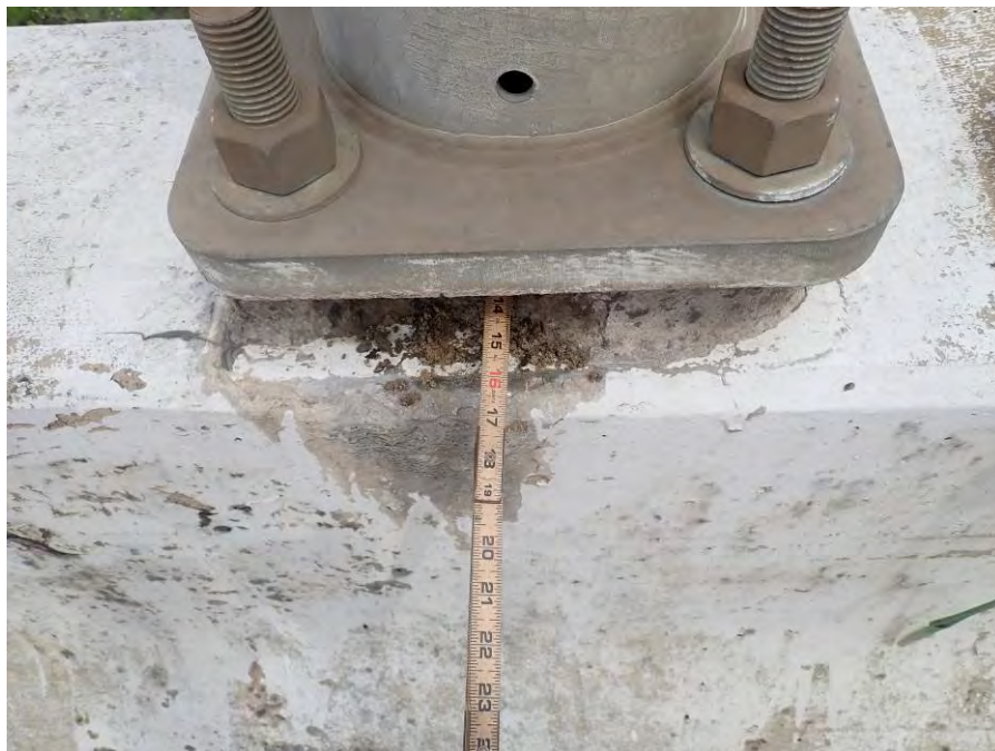
Photograph No. 24 – Hole in Base Mortar Up to 15” Deep in Span 5 at the Support for the Sign Structure at the North Parapet
