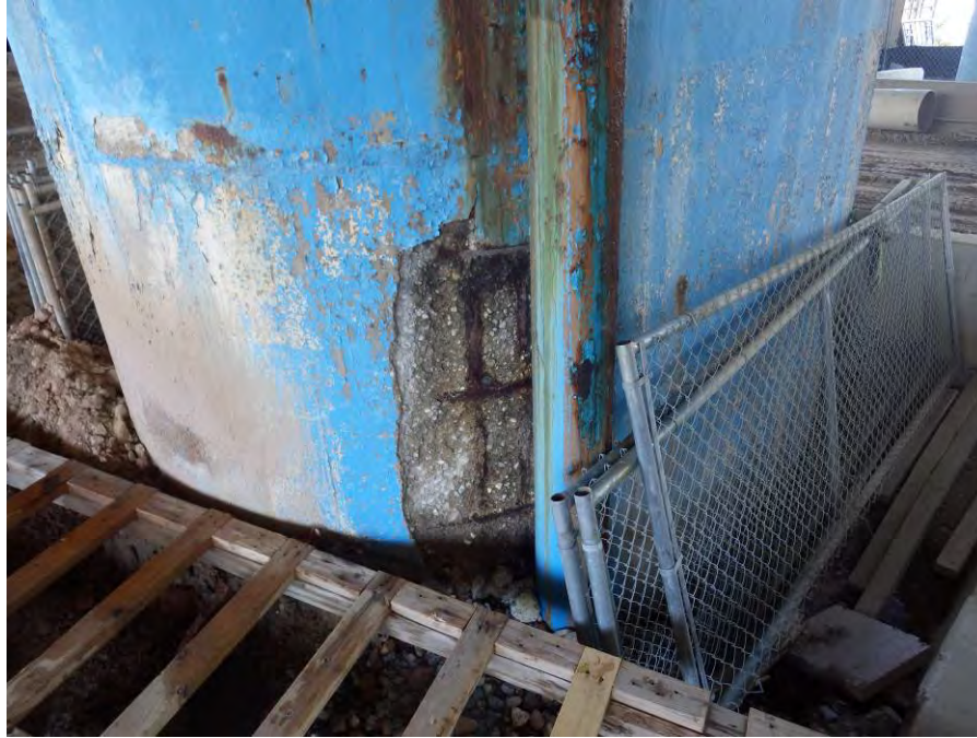
Photograph No. 65 – Bent 4, Column 2, 24” Wide x 6’-0” High x Up to 2 1/2” Deep Spall with Exposed Corroded Reinforcing Steel at the Base of the East Face behind the Drain Pipe
