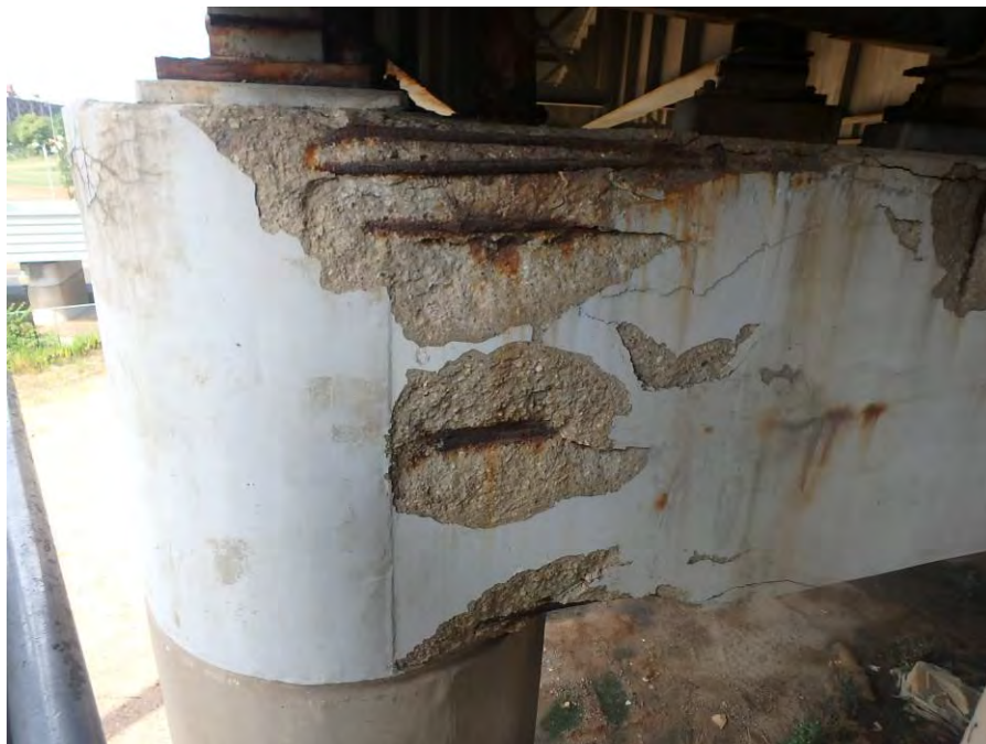
Photograph No. 60 – Spalls with Exposed Corroded Reinforcing Steel in the East Face of the West Pier at the South End
