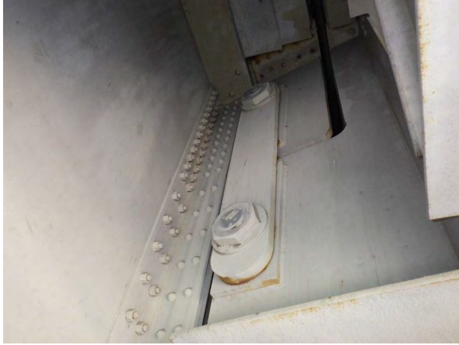
Photograph No. 13 – Typical Pin and Hanger Assembly. Note Areas of Minor Corrosion (North Side of Girder 3 of Span 9 at Bent 9 Shown)
