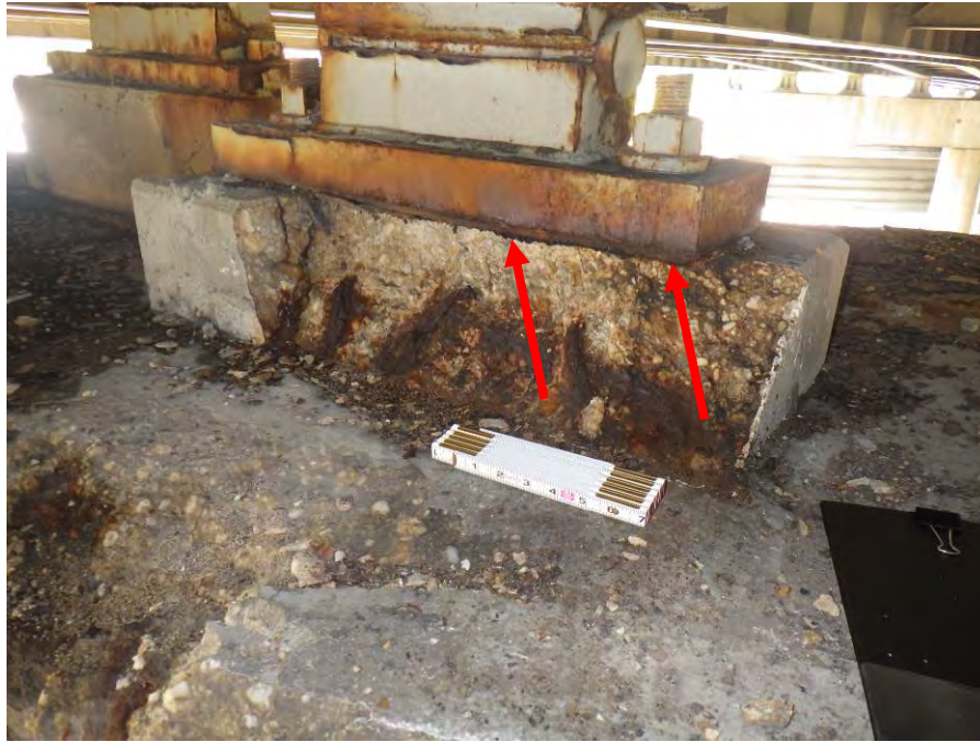
Photograph No. 57 – 23” Long x 6 3/4” High x Up to 5” Deep Spall with Exposed Reinforcing Steel Undermining the Masonry Plate (Arrows) in the Northeast Corner of the Girder 16 Bearing Pedestal at the West Pier
