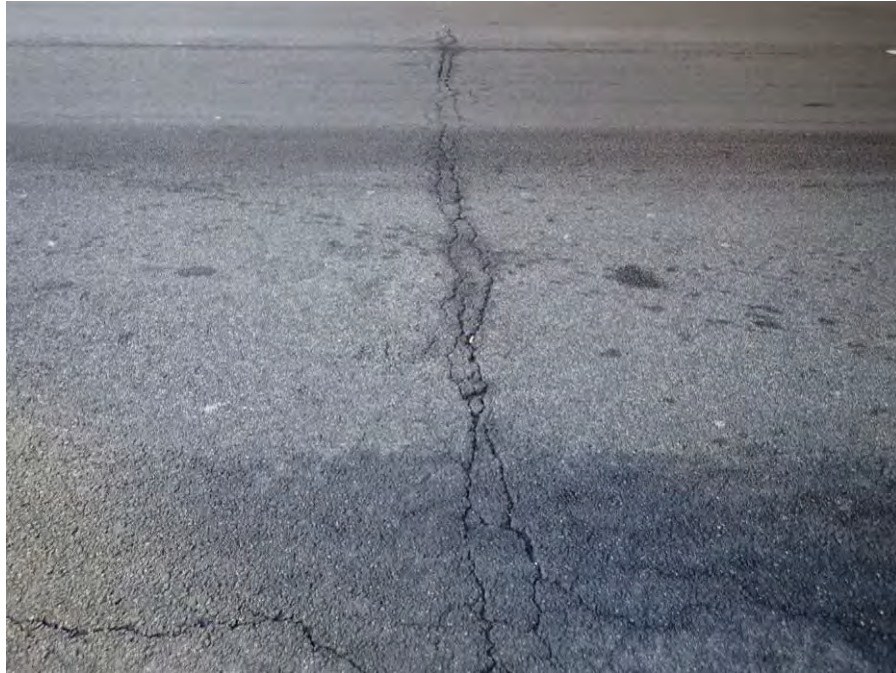
Photograph No. 29 – Up to 1/4" Wide Transverse Crack Spanning the Full-Width of the Roadway at the North End of the Bridge, Looking East
