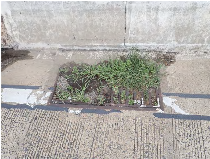
Photograph No. 28 – Westbound Lanes – Broken Drainage Grate in Span 8. Scupper Completely Clogged with Debris
