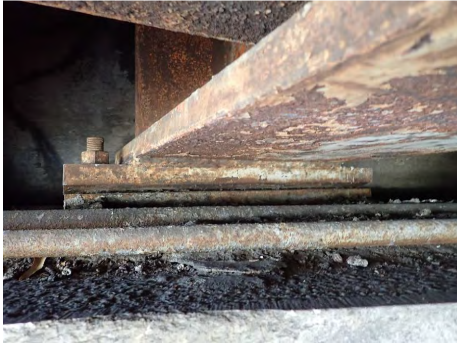
Photograph No. 9 – Typical East Abutment Bearing. Note Deteriorated Paint and Minor Corrosion. Bearing 2 Shown
