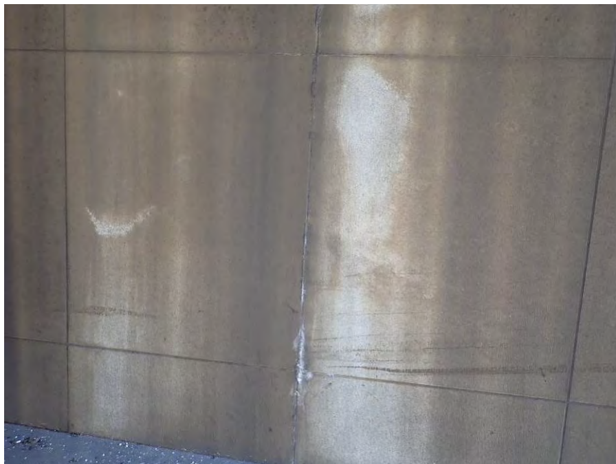
Photograph No. 18 – Cracked Mortar with Efflorescence in the East Abutment Stem
