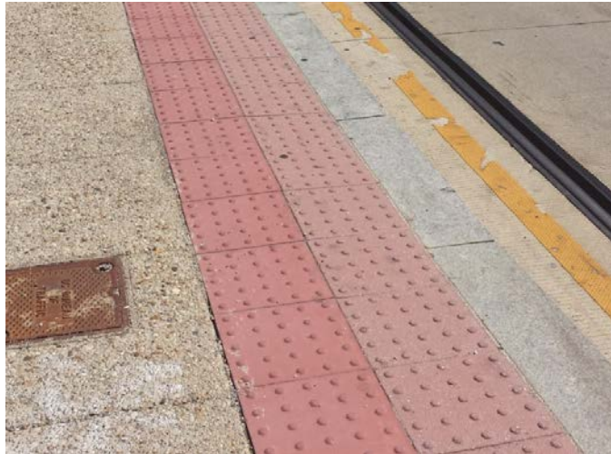
Figure 3-10 | Tactile Platform Warning Strip
