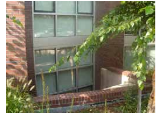
Window wells are a typical example of an areaway that is used to permit light into below-grade residential units.
