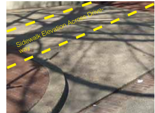
The elevation of the sidewalk where it crosses the driveway should be level with the adjacent sidewalk.
