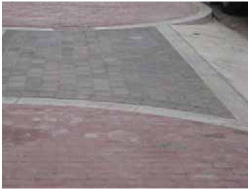
The grade of sidewalks crossing driveways must flush with pavement.
