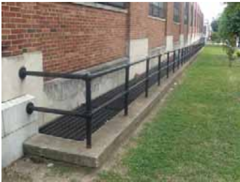
Areaways are used to get light into lower levels of commercial or industrial buildings.
