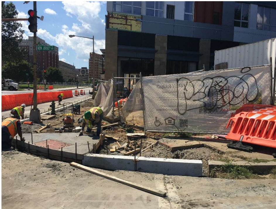
Picture No. 3 - 08/18/2020 – Installation of PCC wheelchair ramp at the intersection of NJ Ave and H St., NW corner (West View)
