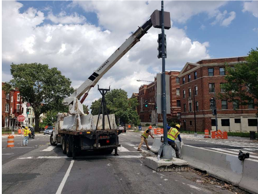
Picture No. 1: 08/17/2020 – Temporary barriers being moved along NY Ave between 1 st St. and NJ Ave. for Phase 4 switch (East View)
