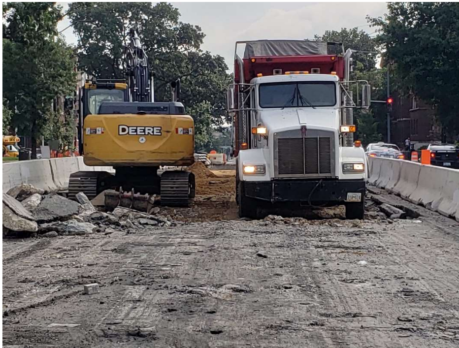
Picture No. 10 – 08/21/2020 – Full depth roadway excavation in progress for Phase 4 along NY Ave between 1 st St. and M St. (East View)
