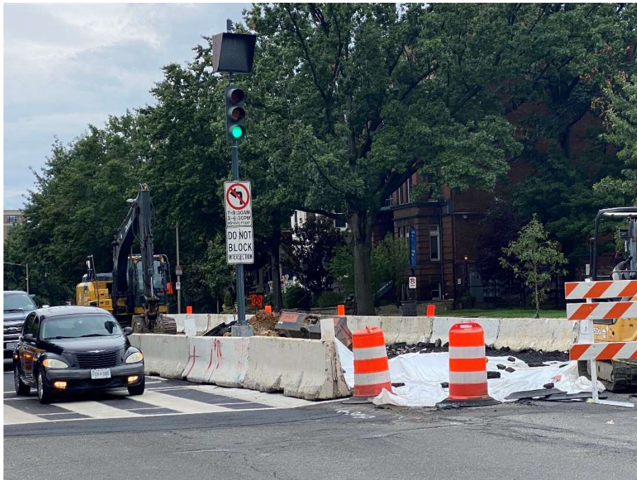
Picture No. 5 – 08/19/2020 – Inspection of MOT at the intersection of NY Ave and NJ Ave. (East View)
