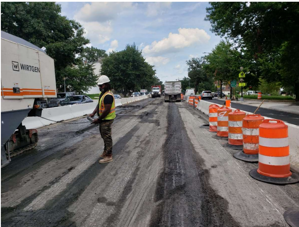
08/20/2020 – Pavement milling in progress along Phase 4 of NY Ave between 1 st St. and NJ Ave St. (East View)
