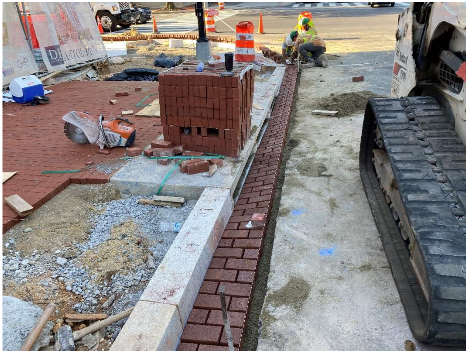
Picture No. 6 – 08/20/2020 – Installation of brick gutter in progress at NE corner of 2 nd St. and H St. (South View)
