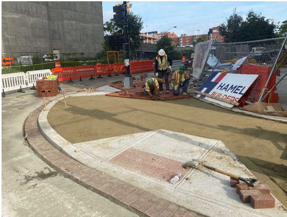
Picture No. 9 – 08/21/2020 – Brick sidewalk being installed at the NE corner of the intersection of H St. and 2 nd St. (North View)
