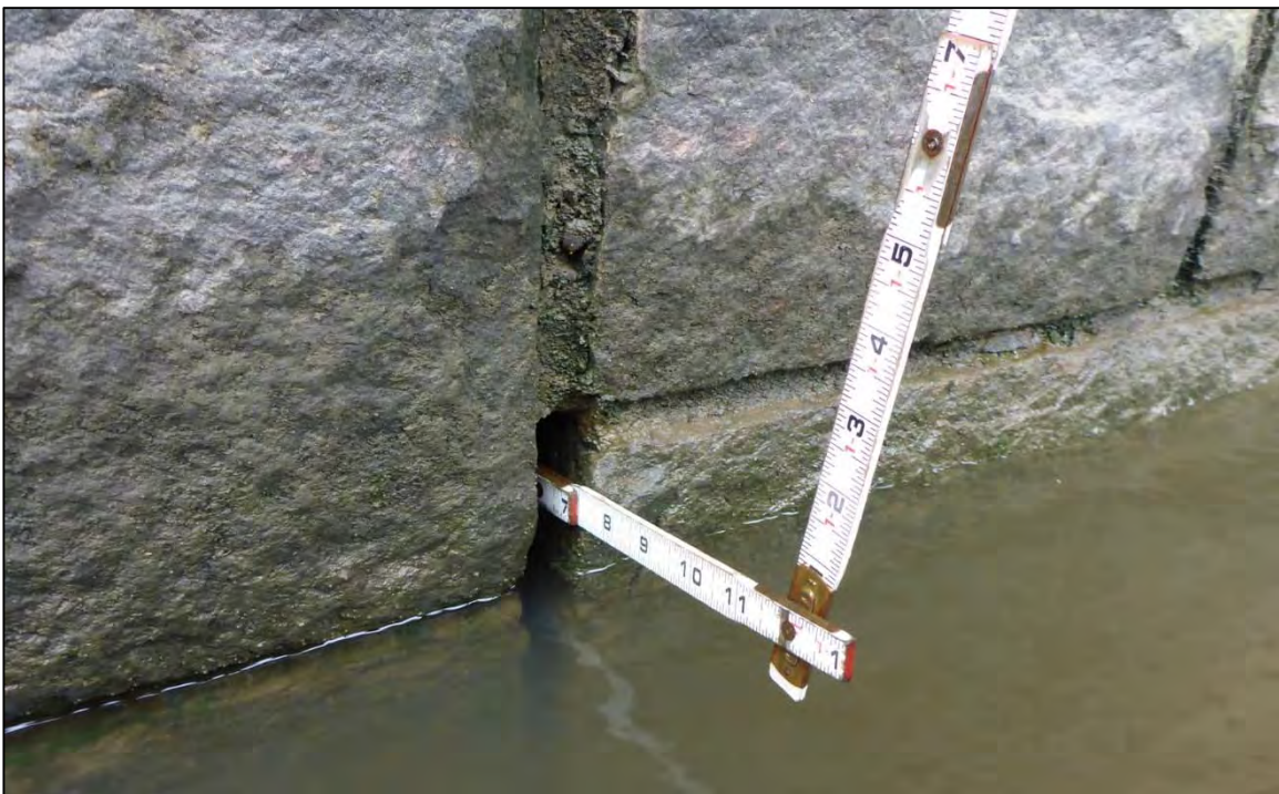
Photograph 12: View of Mortar Loss at Pier 3 Upstream Nose, Looking East
