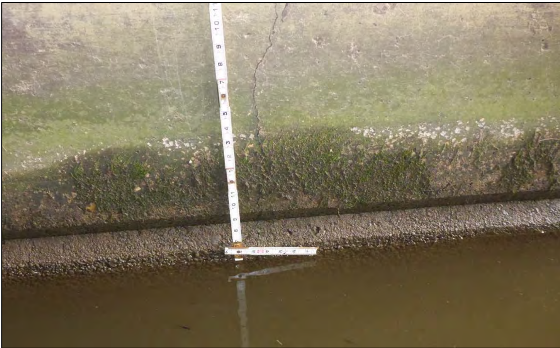
Photograph 6: View of Typical Crack Extending from Mudline to Top of Pier 1, Looking West
