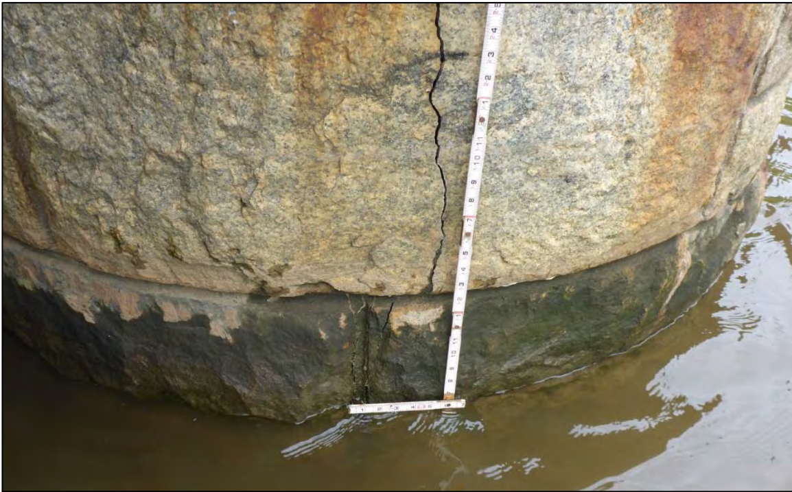
Photograph 5: View of Vertical Crack in Fascia Stones on Pier 1 Upstream Nose, Looking South
