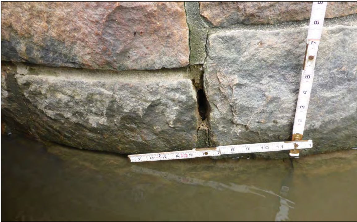
Photograph 11: View of Mortar Loss at Pier 3 Downstream Nose, Looking North
