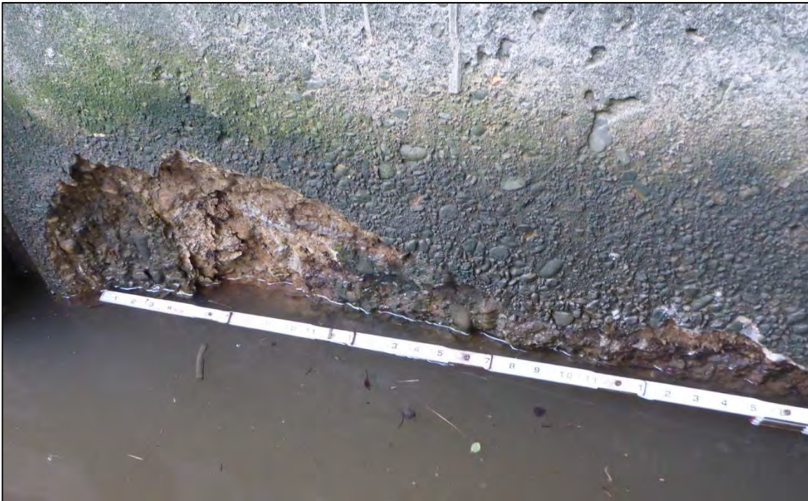
Photograph 15: View of Typical Scale on East Abutment, Looking East
