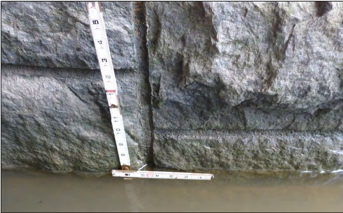
Photograph 9: View of Typical Fascia Stone Mortar Loss at Pier 2 Southwest Face, Looking East
