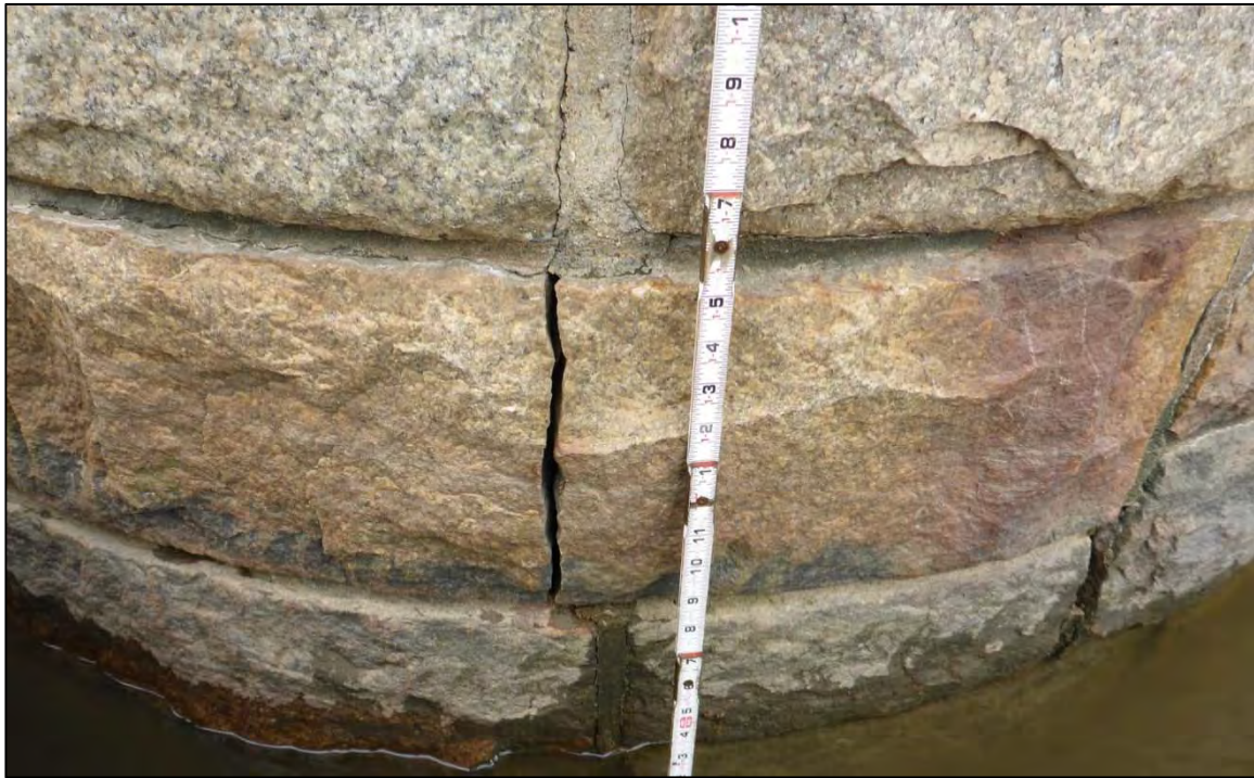
Photograph 13: View of 1/4" Wide Vertical Crack in Fascia Stones at Pier 3 Upstream Nose, Looking South
