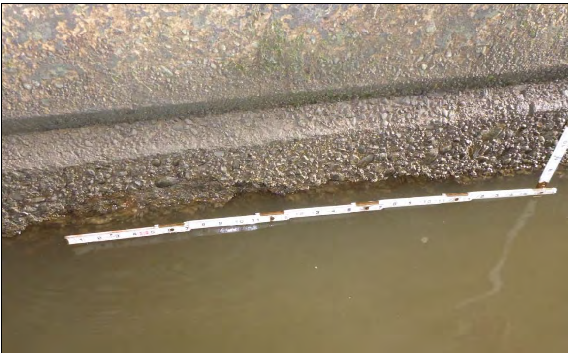
Photograph 8: View of Typical Scale on Pier 2 West Face, Looking East
