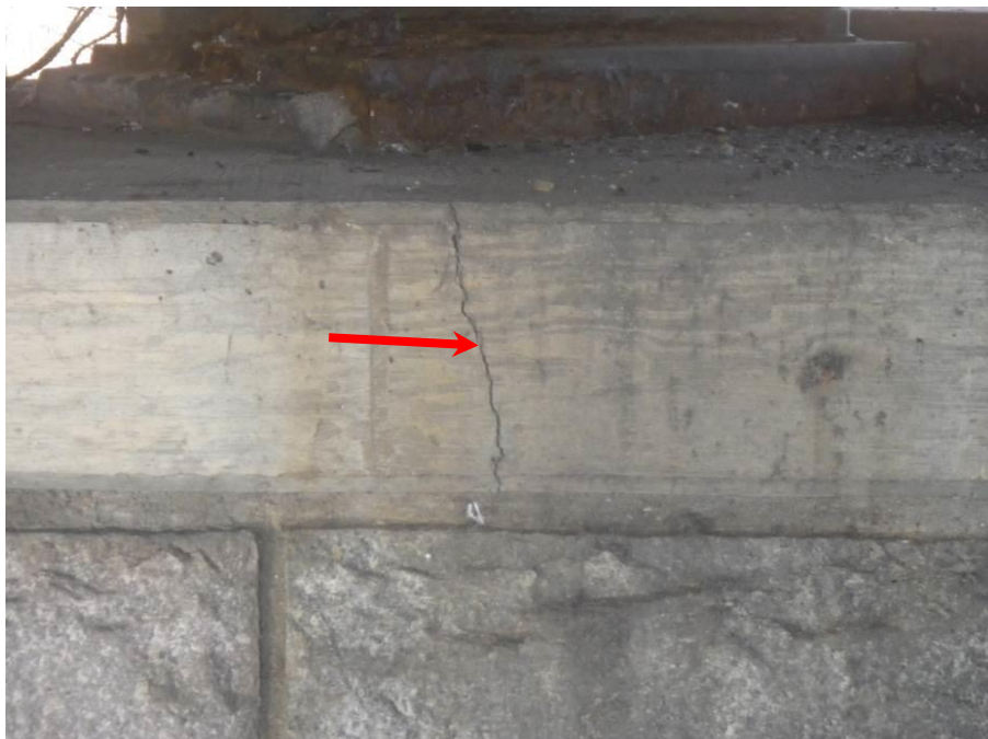
Photograph No. 52 – 1/8" Wide Crack in the East Face of the Pier 1 Cap at Girder 2 (Arrow)
