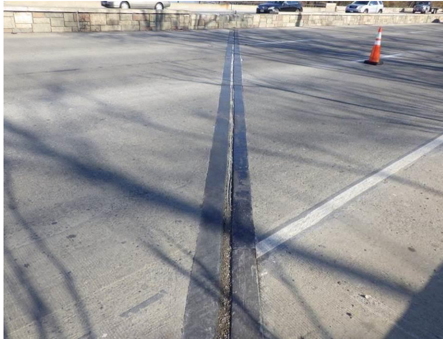
Photograph No. 25 – Compression Joint over Southern Portion of East Abutment, Looking North
