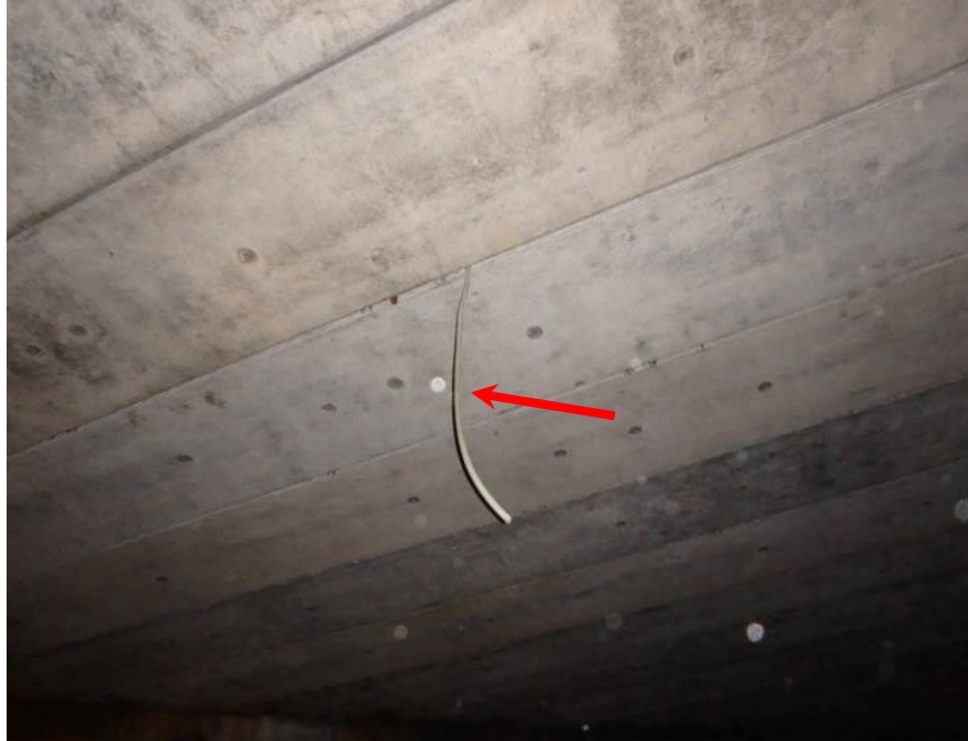
Photograph No. 31 – Joint Material Hanging from between Box Girders in East Abutment Span (Arrow)
