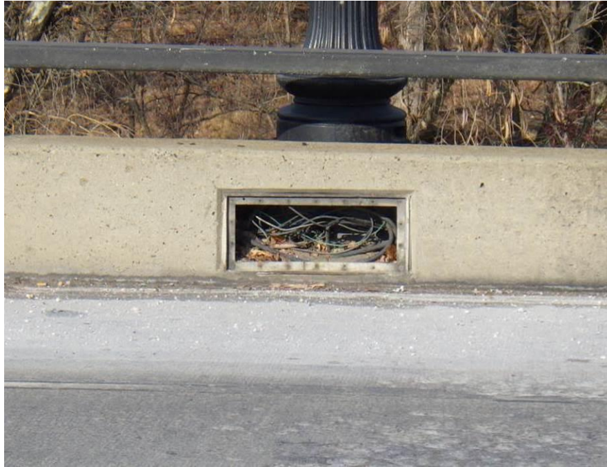
Photograph No. 85 – Missing Junction Box Cover with Exposed Wires in the North Parapet of Span 2
