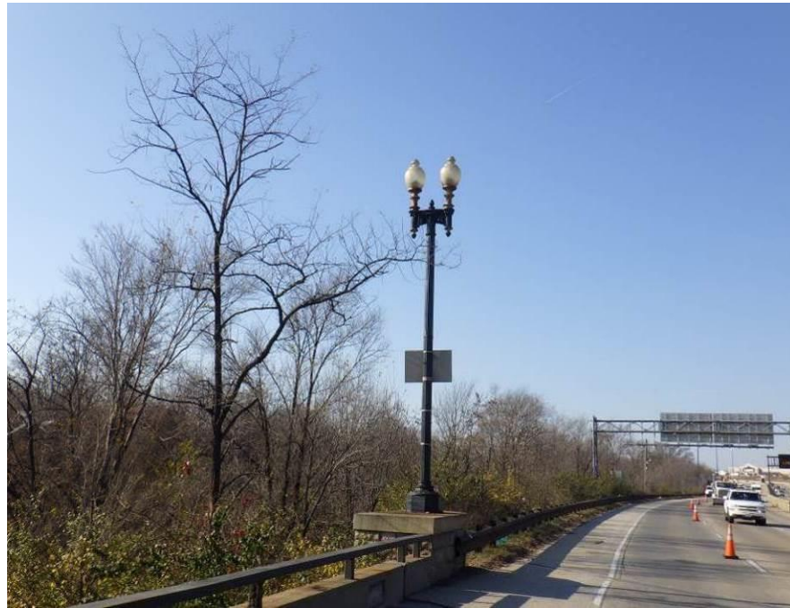
Photograph No. 81 – Typical Double Luminaire Light Standard, Southwest Corner of the Bridge Shown
