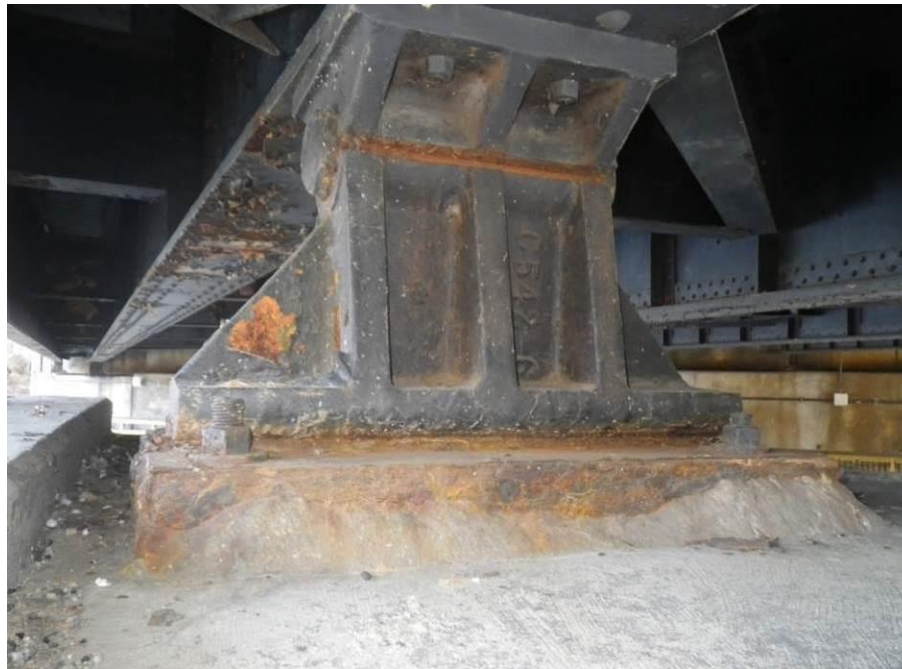
Photograph No. 38 – Moderate Crevice Corrosion between Rocker Bearing and Masonry Plate, Bearing 2, West Face at Pier 3 Shown
