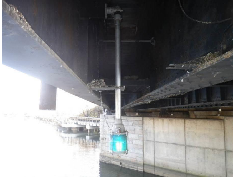
Photograph No. 79 – Replaced Green Navigation Light for the North Side of Span 3
