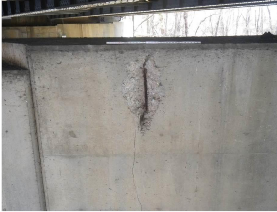
Photograph No. 57 – 2'-4" x 15" x 3 1/2" Deep Spall with Exposed Reinforcing Steel in West Face of Pier 3
