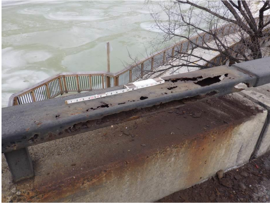
Photograph No. 21 – Areas of 100% Section Loss (Holes) in the East End of the North Bridge Railing
