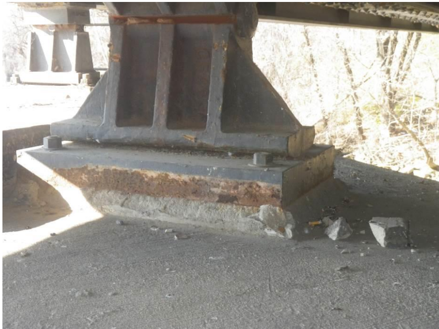
Photograph No. 40 – Spalled Bearing Pedestal Encasement for Girder 7 at Pier 1, Looking Southwest
