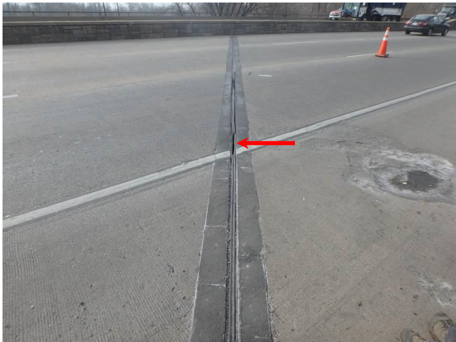
Photograph No. 22 – Compression Joint over Northern Portion of West Abutment, Looking South. Note 2'-6" Long Tear in Joint Material in Right Westbound Lane (Arrow)
