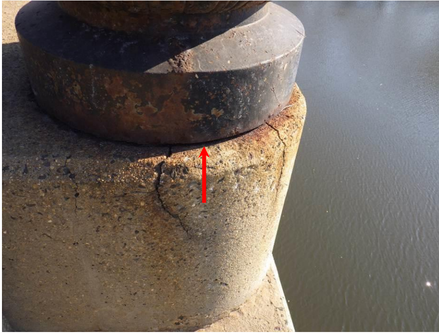
Photograph No. 83 – 1/4" Wide Gap at Bottom of Light Standard and Cracks in Base Concrete, South Light Standard in Span 2 Shown (Arrow)
