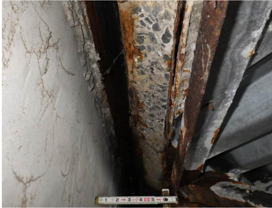
Photograph No. 17 – 26'-0" Long x 3" Wide x 6" Deep Spall in the Soffit at the West Abutment adjacent to the S.I.P. Forms, Looking North
