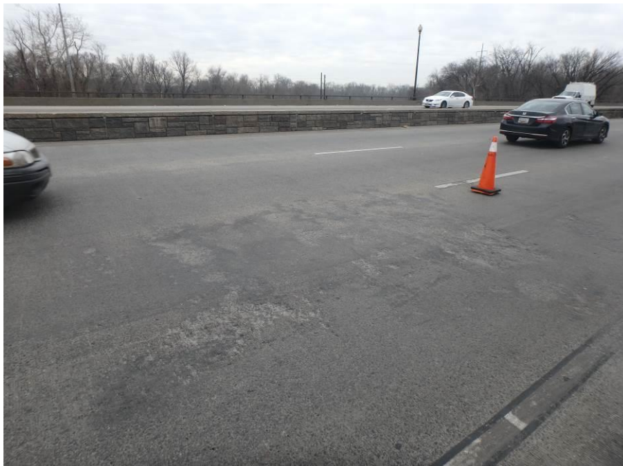
Photograph No. 14 – 12'-0" Long x 6'-0" Wide Area of Shallow Spalling in the Right Westbound Lane of Span 2
