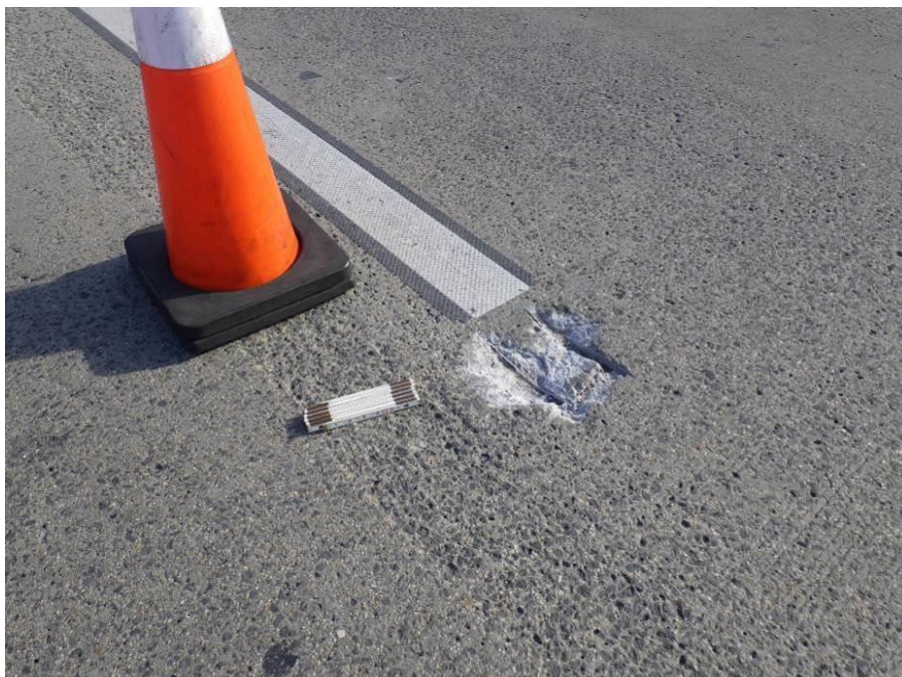
Photograph No. 16 – Missing Roadway Reflector between the Left and Center Eastbound Lanes
