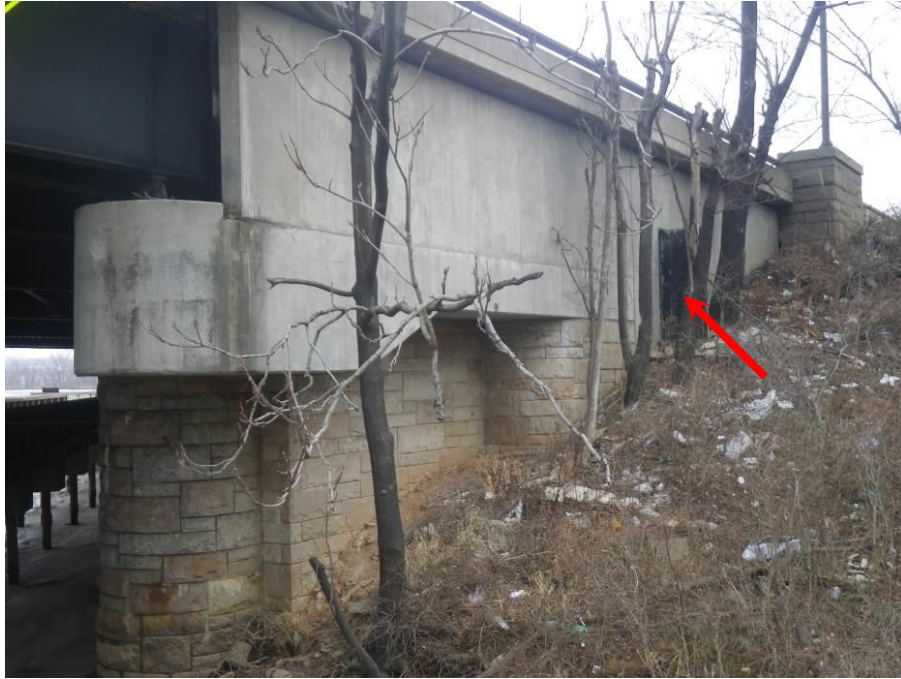
Photograph No. 67 – Southeast Curtain Wall. Note Vegetation Growth adjacent to Exterior of Curtain Wall and Access Door to East Abutment Span (Arrow)
