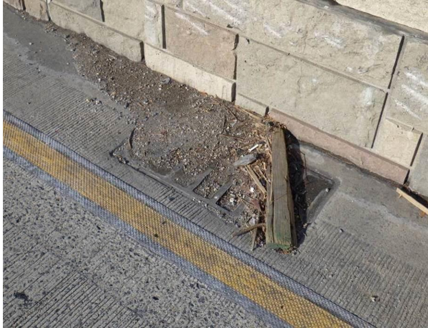
Photograph No. 29 – 100% Clogged Scupper, Span 1 Scupper at Median Shown
