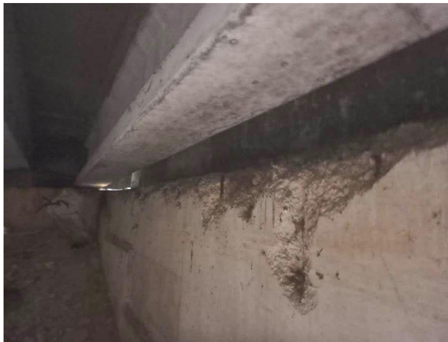
Photograph No. 64 – Spalling along the Top Interior Side of the South Curtain Wall in the East Abutment Span
