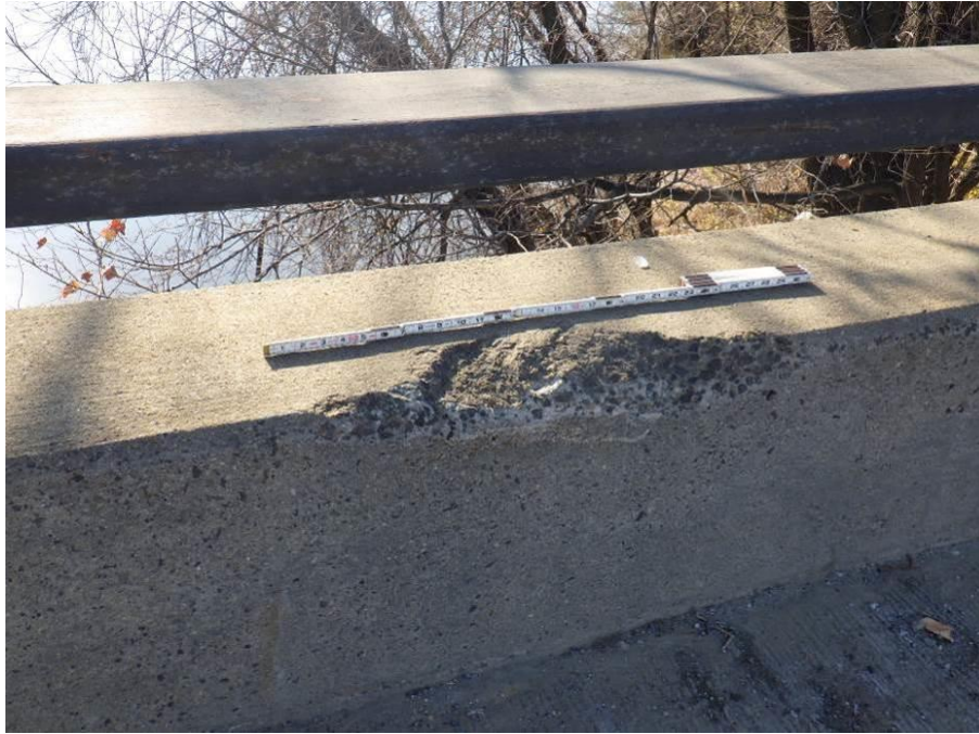
Photograph No. 19 – 2'-4" Long x 3" x 3" Spall in Upper North Corner of South Parapet
