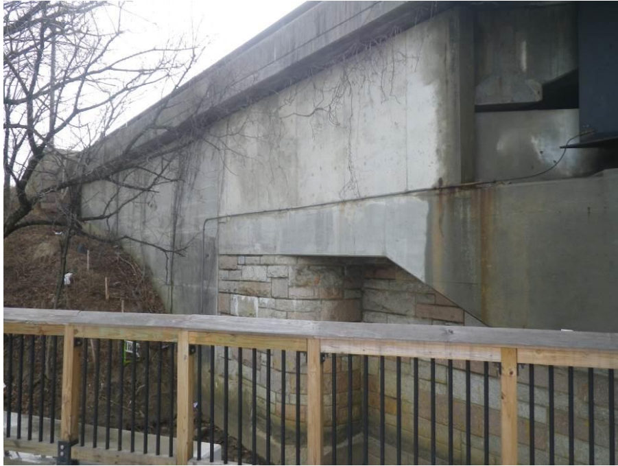
Photograph No. 65 – Northeast Curtain Wall, Minor Vegetation Growth adjacent to Exterior of Curtain Wall
