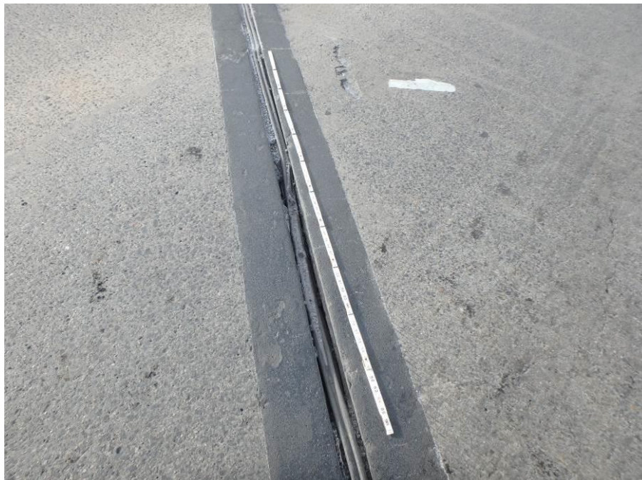
Photograph No. 26 – Compression Joint over Northern Portion of West Abutment, Damaged and Depressed Joint Material in the Right Westbound Lane
