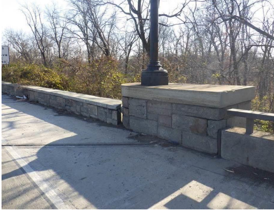
Photograph No. 75 – Southeast Transition to Masonry Railing on East Approach, Looking Southeast
