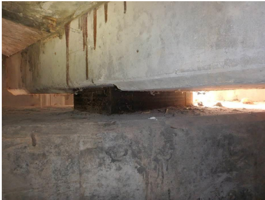
Photograph No. 36 – Typical Elastomeric Bearing Pad for Concrete Box Girders, Beam 20 at the West Abutment Shown, Looking Southeast
