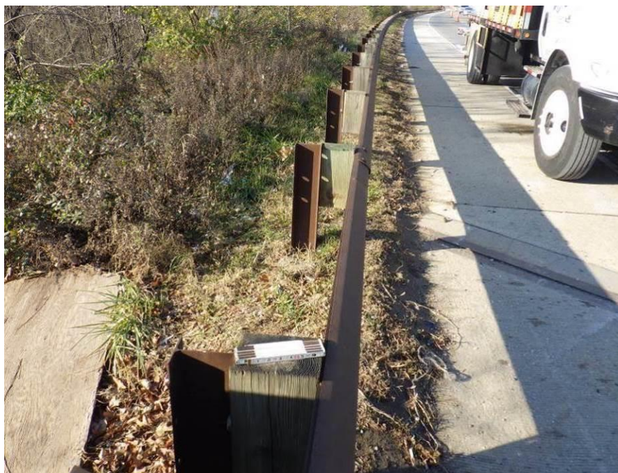
Photograph No. 78 – Southwest Guide Rail not Properly Stiffened at the Bridge, Looking West
