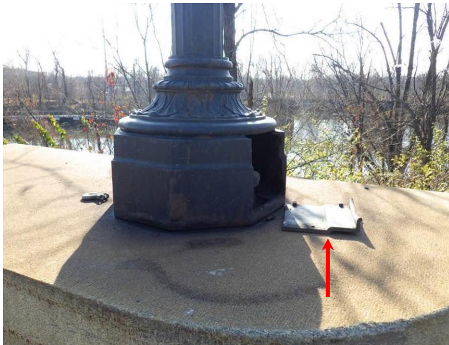
Photograph No. 84 – Displaced Access Panel for the Southwest Light Standard Base Exposing Wires (Arrow)
