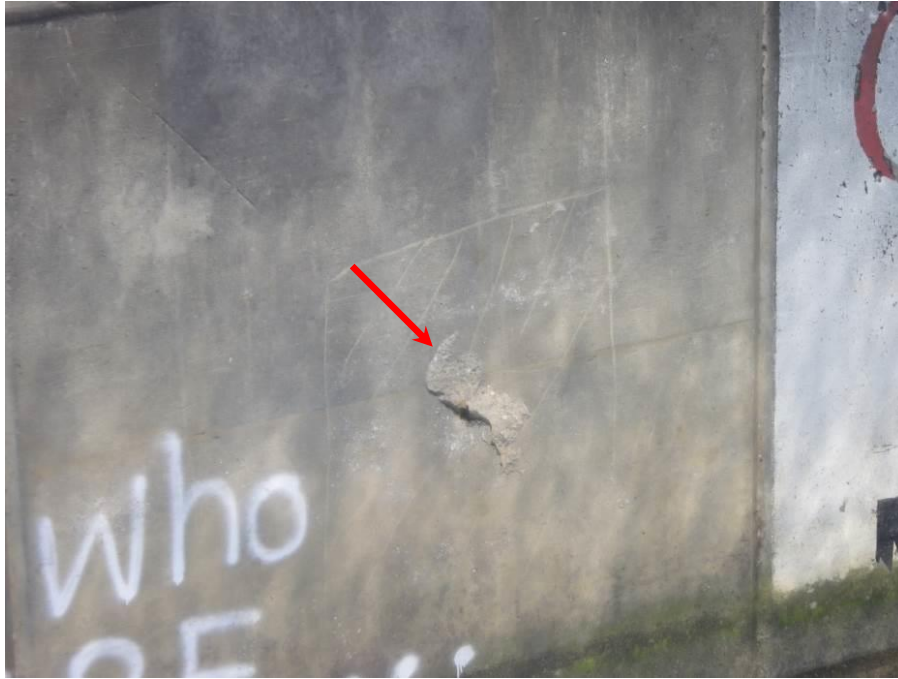
Photograph No. 53 – 13” Long x 16” High x Up to 1 3/4” Deep Spall inside of a 3’-0” Long x 4’-4” High Unsound Area in the East Face of Pier 1 below Girder 5
