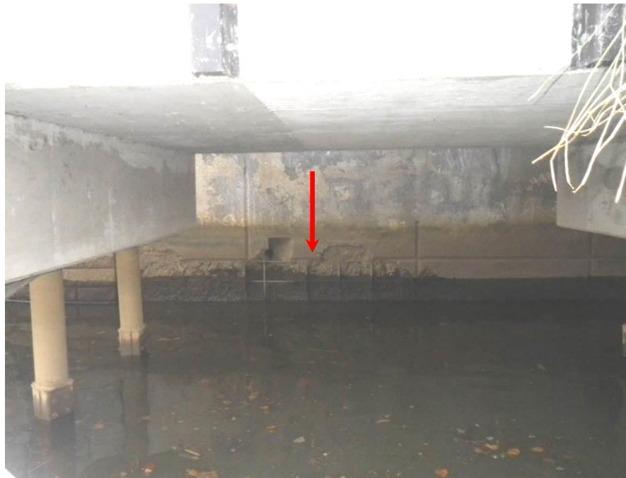
Photograph No. 46 – Typical Severe Scaling with Exposed Reinforcing Steel below Waterline at East Abutment, Visible Due to Low Tide (Arrow)
