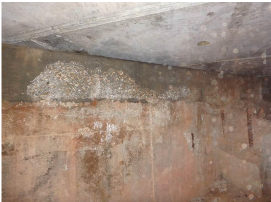
Photograph No. 60 – Spalls and Unsound Concrete in the East Abutment Grade Beam below Box Beam 12, Looking Southeast
