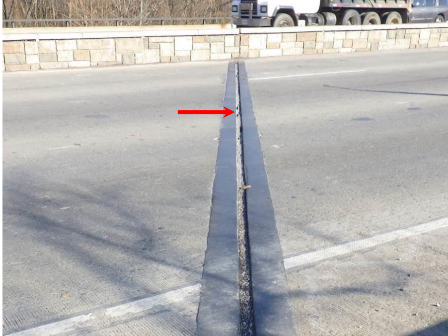
Photograph No. 23 – Compression Joint over Southern Portion of West Abutment, Looking North. Note Debonded Sections of Joint Material (Arrow)
