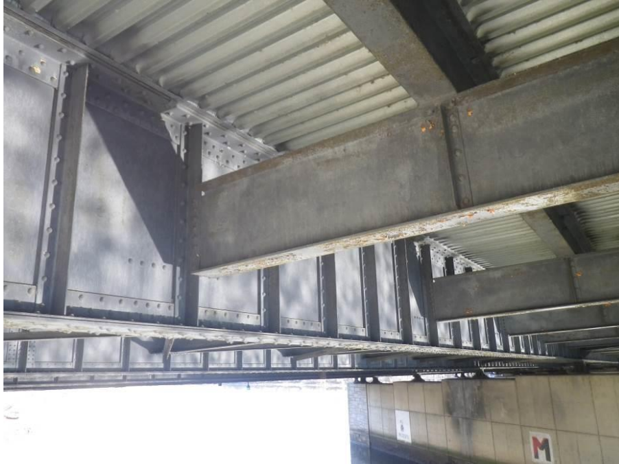
Photograph No. 35 – Typical Floorbeam Connections in Good Condition with Minor Paint Deterioration, Girder 6 in Span 2 Shown, Looking Northeast
