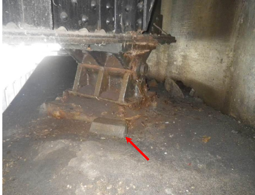
Photograph No. 37 – Typical Rocker Bearing with Minor Paint Deterioration and Surface Corrosion at Base, East Abutment Bearing 3 Shown. Note Spalled Concrete Pedestal Plate Encasement (Arrow)
