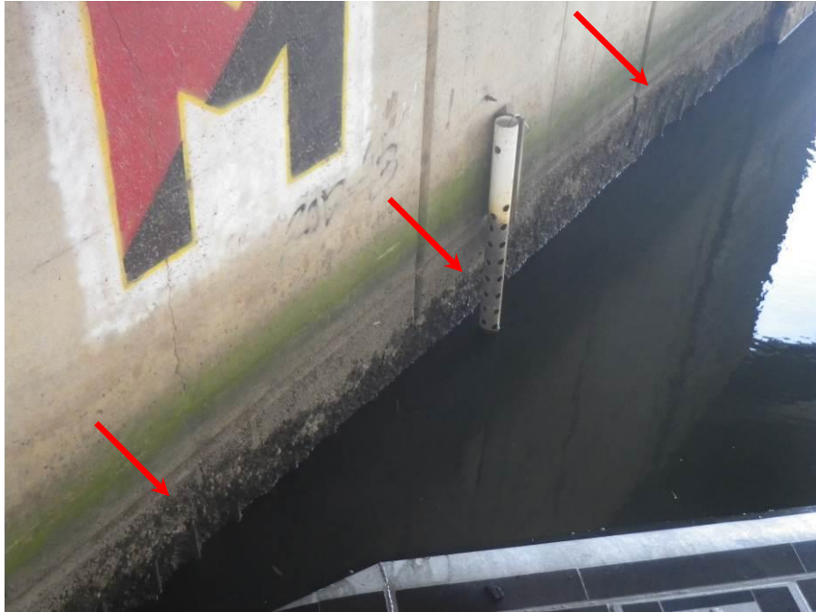
Photograph No. 47 – Typical Severe Scaling with Exposed Reinforcing Steel below Waterline at West Face of Pier 2, Visible Due to Low Tide (Arrows)
