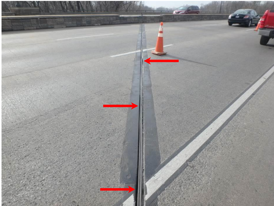
Photograph No. 24 – Compression Joint over Northern Portion of East Abutment, Looking South. Note Debonded Sections of Joint Material (Arrows)
