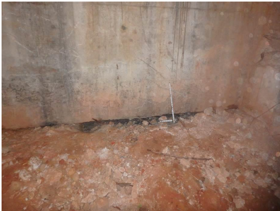
Photograph No. 61 – 6'-0" Long x 2'-8" Deep Area of Minor Erosion below the Grade Beam below Box Beam 4, Looking East
