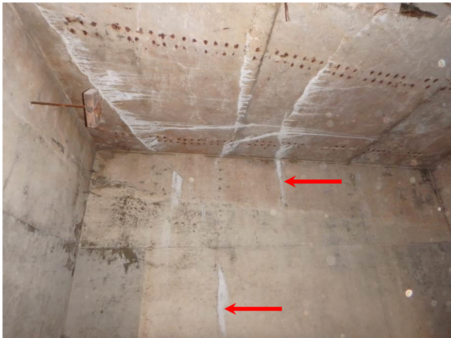
Photograph No. 58 – Typical Full-height Vertical Hairline Cracks with Efflorescence in the East Face of the East Abutment Stem, between Beams 13 and 14 Shown, Looking West (Arrows)
