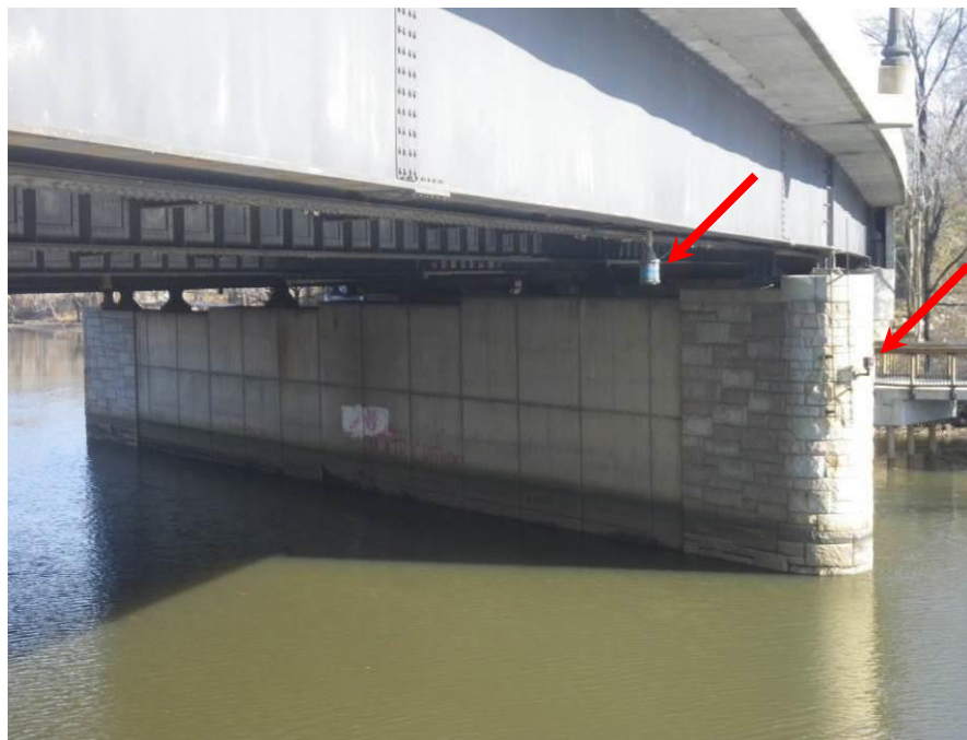
Photograph No. 44 – Pier 3, West Face. Note Non-Functioning Navigation Lights on South Side of Bridge (Arrows)
