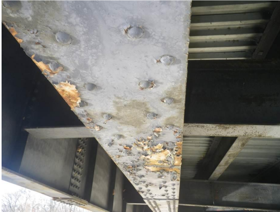
Photograph No. 33 – Typical Peeling Paint on Girder Bottom Flanges, Girder 7 in Span 2 near Pier 1 Shown, Looking Southwest
