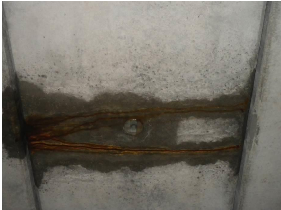
Photograph No. 30 – Evidence of Moisture Leaking between Box Girders 12 and 13 in West Abutment Span
