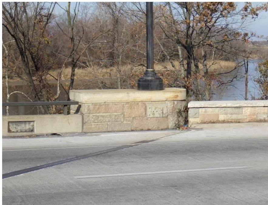
Photograph No. 74 – Northeast Transition to Masonry Railing on East Approach, Looking North
