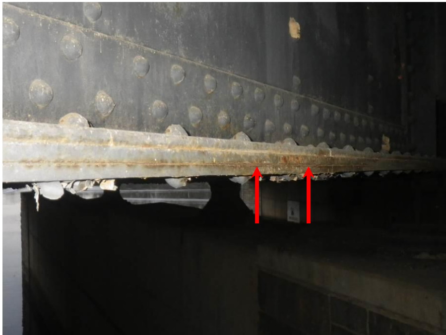
Photograph No. 34 – Girder 7, Span 1, Pier 1, South Face, 1/8" Thick Crevice Corrosion between Bottom Flange Cover Plates (Arrows)
