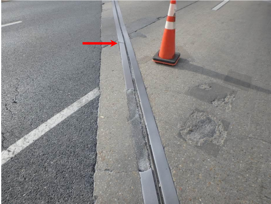
Photograph No. 73 – Asphaltic Material in Place of a Section of Metal Joint Armor for the East Approach Joint in the Right Westbound Lane, Looking Southwest. Note adjacent Broken Section of Joint Armor (Arrow)
