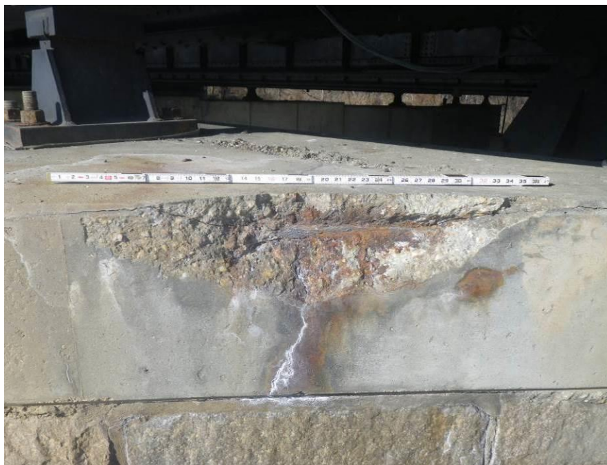
Photograph No. 54 – 2’-8” Wide x 6 1/2” High x Up to 3” Deep Spall with Exposed Corroded Reinforcing Steel and Efflorescence in East Face of Pier 2
