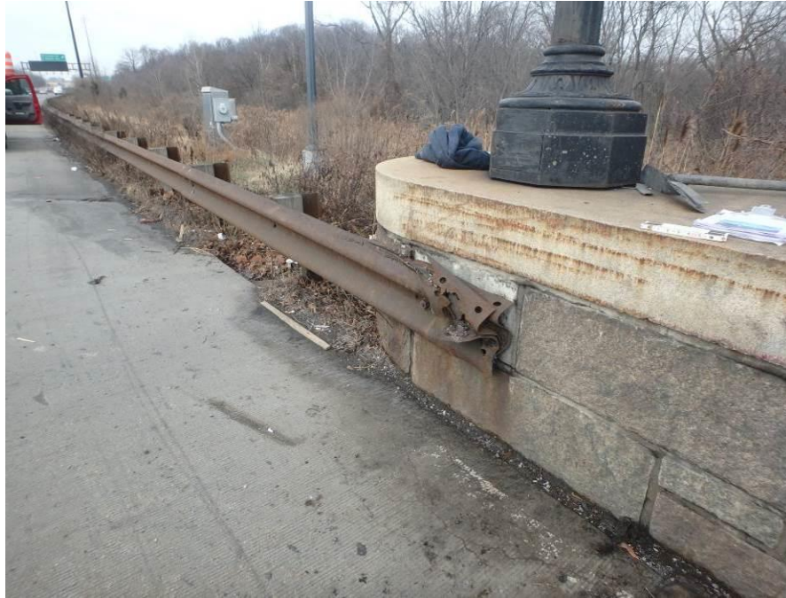
Photograph No. 77 – Non-Standard Attachment of Northwest Guide Rail to Bridge Railing. Note Impact Damage
