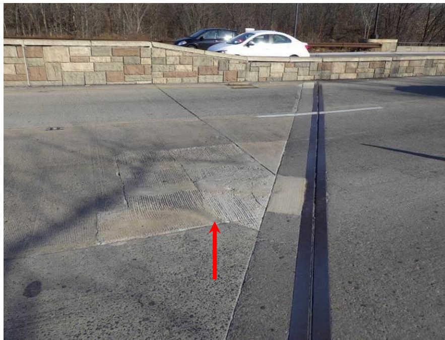
Photograph No. 70 – New Concrete Patch in the Center Eastbound Lane of the West Approach Roadway (Arrow)
