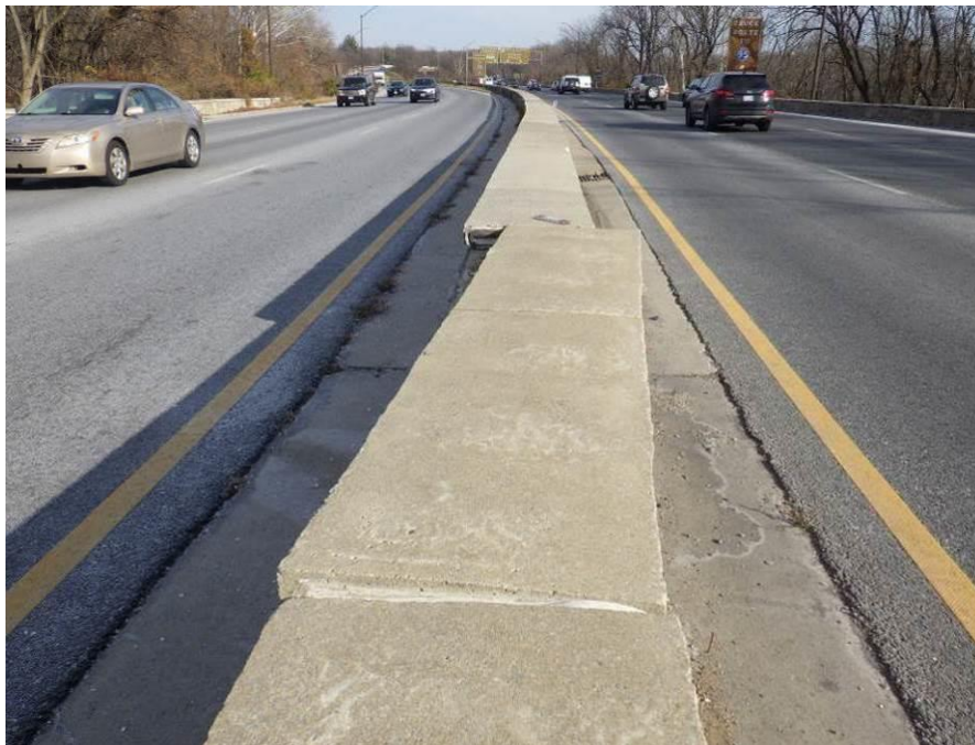
Photograph No. 76 – 10' Long Section of the East Approach Median Capstone Loose and Displaced Up to 9" to the South, Looking East
