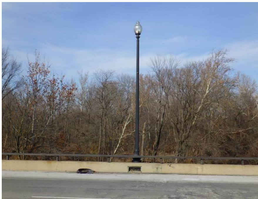
Photograph No. 82 – Typical Single Luminaire Light Standard. Replaced Light Standard on the North Side of Span 2 Shown
