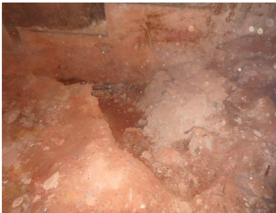
Photograph No. 62 – 11'-0" Long x 8'-6" Wide x Up to 4'-0" Deep Erosion Hole in the East Abutment Span, Looking North
