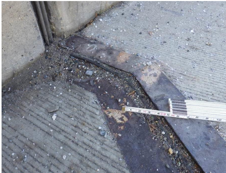
Photograph No. 28 – 3/4" Vertical Differential of the Joint Armor and Bulging Joint Material in South Shoulder at the Far End of the West Abutment Span in the Eastbound Lanes, Looking Southwest
