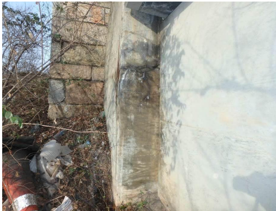
Photograph No. 50 – Hairline Cracks with Efflorescence and Corrosion Staining at the Southeast Corner of the West Abutment Grade Beam
