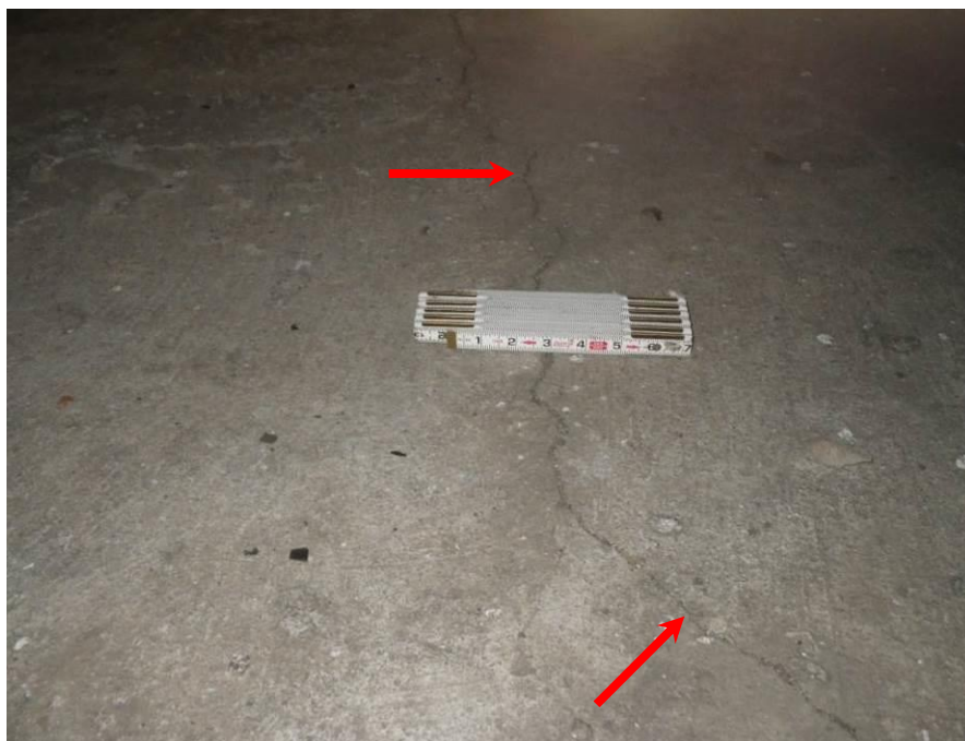
Photograph No. 56 – Hairline to 1/8" Wide Crack Extending across Pier Cap from Vertical Crack in Stem (Arrows), Pier 3 between Girders 3 and 4 Shown
