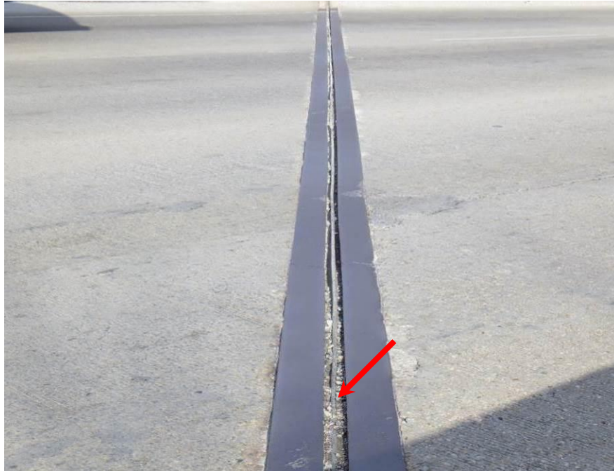
Photograph No. 27 – Typical Strip Seal Joint at the Far End of the Abutment Spans, North Portion of East Joint Shown. Note Moderate Debris at Shoulder (Arrow)
