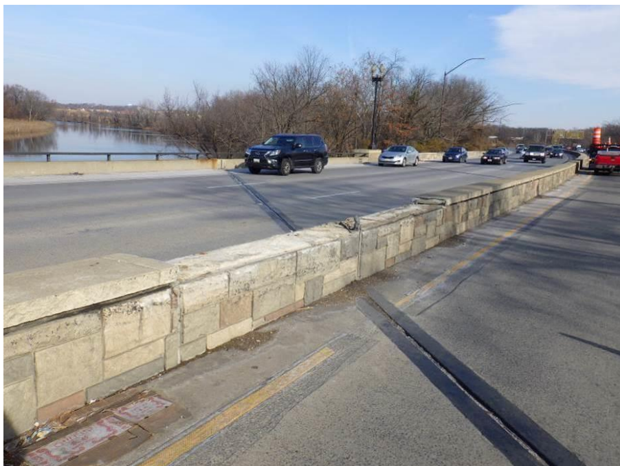
Photograph No. 20 – 19'-0" Long Section of Missing Median Barrier Capstone at the East End of the Bridge
