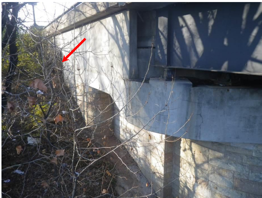
Photograph No. 68 – Southwest Curtain Wall. Note Vegetation Growth adjacent to Exterior of Curtain Wall and Access Door to West Abutment Span (Arrow)
