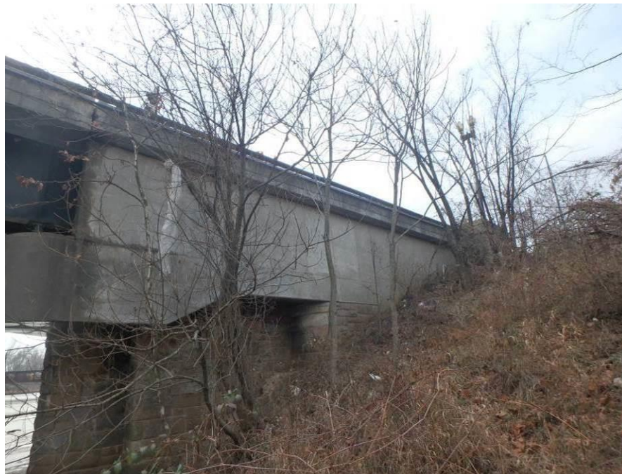
Photograph No. 66 – Northwest Curtain Wall. Note Minor Vegetation Growth adjacent to Exterior of Curtain Wall
