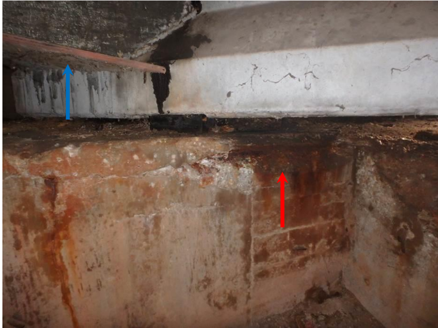
Photograph No. 59 – South End of the East Abutment Grade Beam, 24” Long x 5” High x 2” Deep Spall with Exposed Corroded Reinforcing Steel (Red Arrow). Note Remaining Plywood Formwork (Blue Arrow), Looking Southeast
