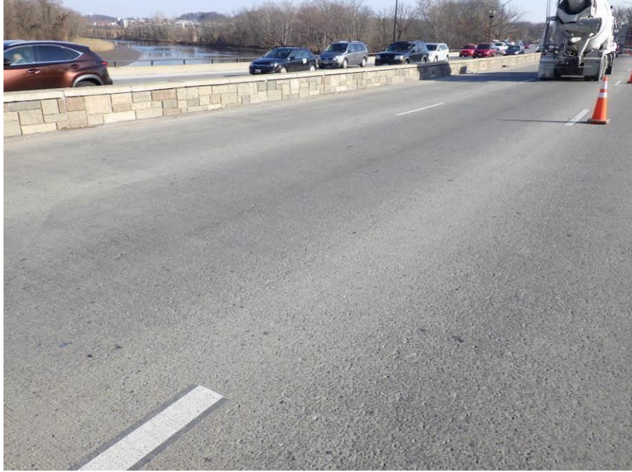
Photograph No. 13 – Typical Wearing Surface, Eastbound Lanes in Spans 2 and 3 Shown, Looking Northeast
