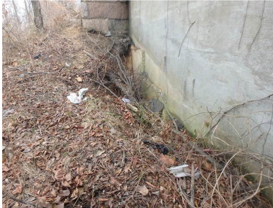
Photograph No. 63 – 12'-0" Long x 4'-0" Wide x Up to 5'-0" Deep Erosion Hole adjacent to the Northeast Wingwall
