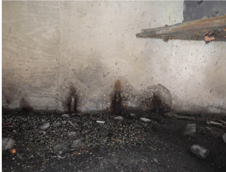
Photograph No. 51 – Three Up to 11" Diameter Spalls with Exposed Corroded Reinforcing Steel in the West Abutment Backwall between Girders 2 and 3
