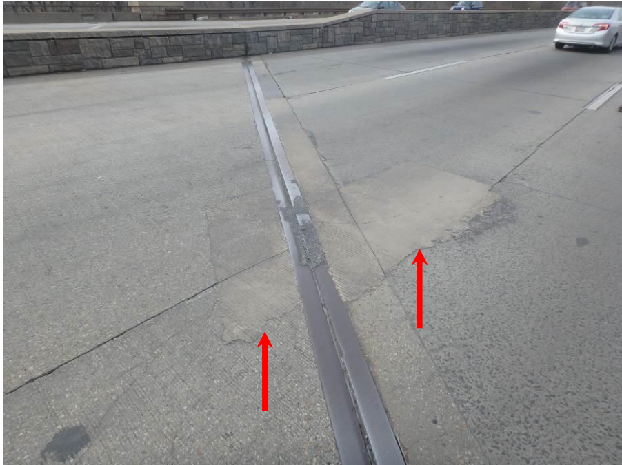
Photograph No. 69 – New Concrete Patch in the Center Westbound Lane of the West Approach Slab and West Approach Roadway (Arrows)
