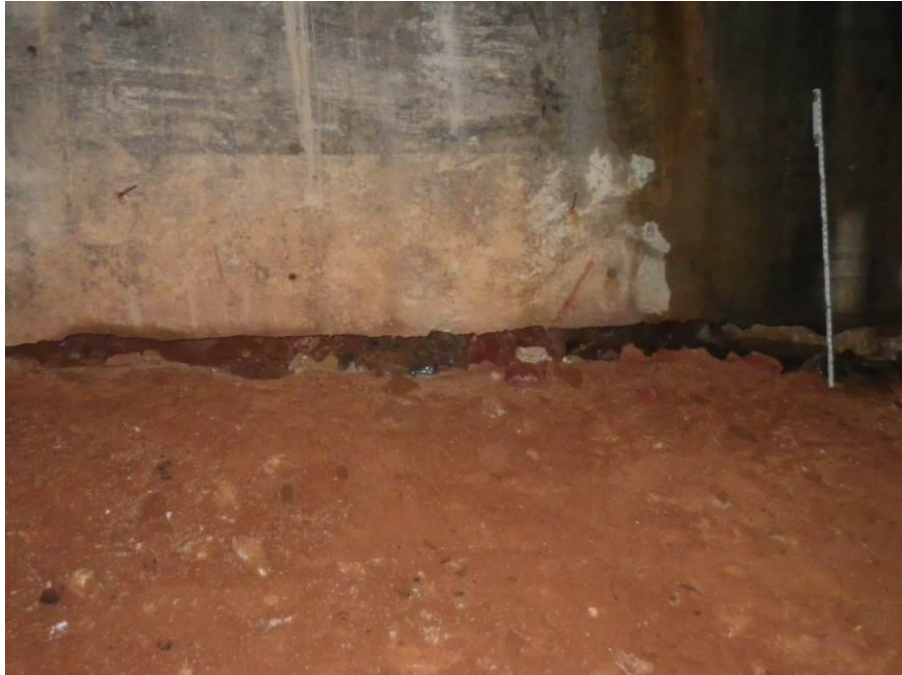
Photograph No. 49 – Settlement of West Abutment Span Fill Material along Base of West Abutment Grade Beam Allowing Various Sizes of Voids
