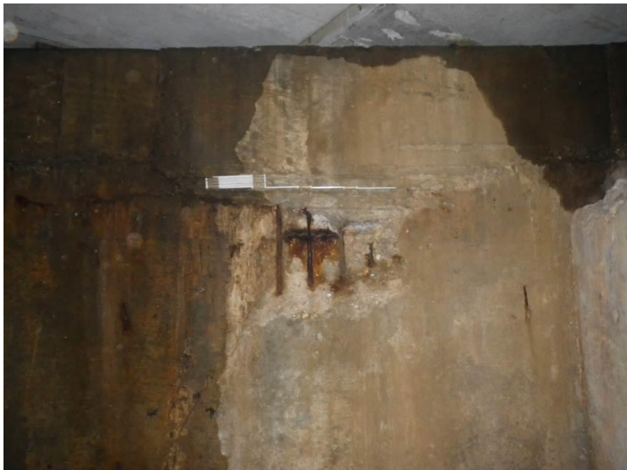
Photograph No. 48 – 22" x 17" x 2 1/8" Deep Spall with Up to 75% Section Loss of Exposed Corroded Reinforcing Steel in West Abutment Grade Beam between Box Beams 5 and 6, Looking West
